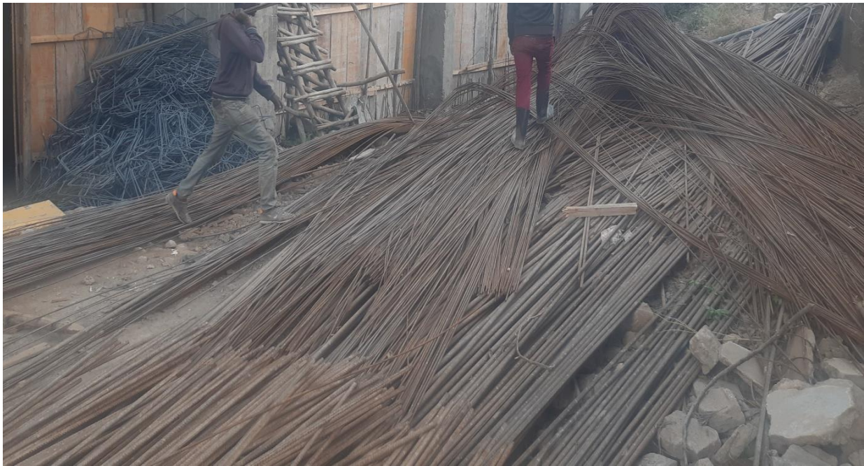
Figure 8: Improper rebar storage on the pathway
