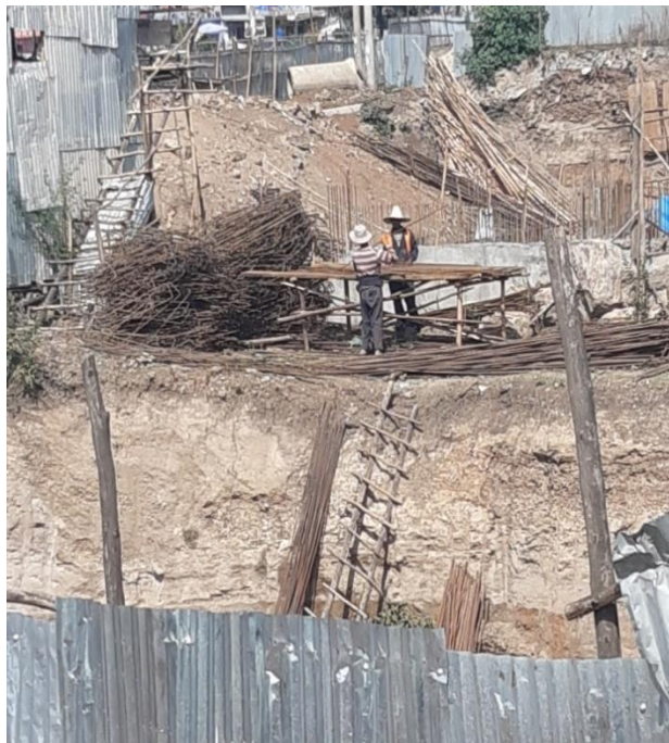
Poor working environment and safety
