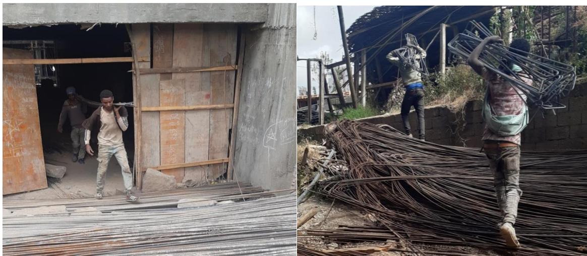
Figure 11: Laborers working on uneven condition
