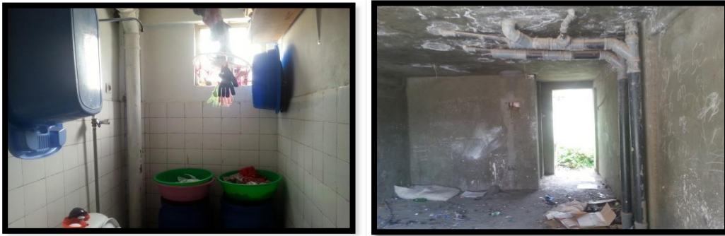
Figure 10: Water and sanitation problem in Ajamba Condominium (new site)
