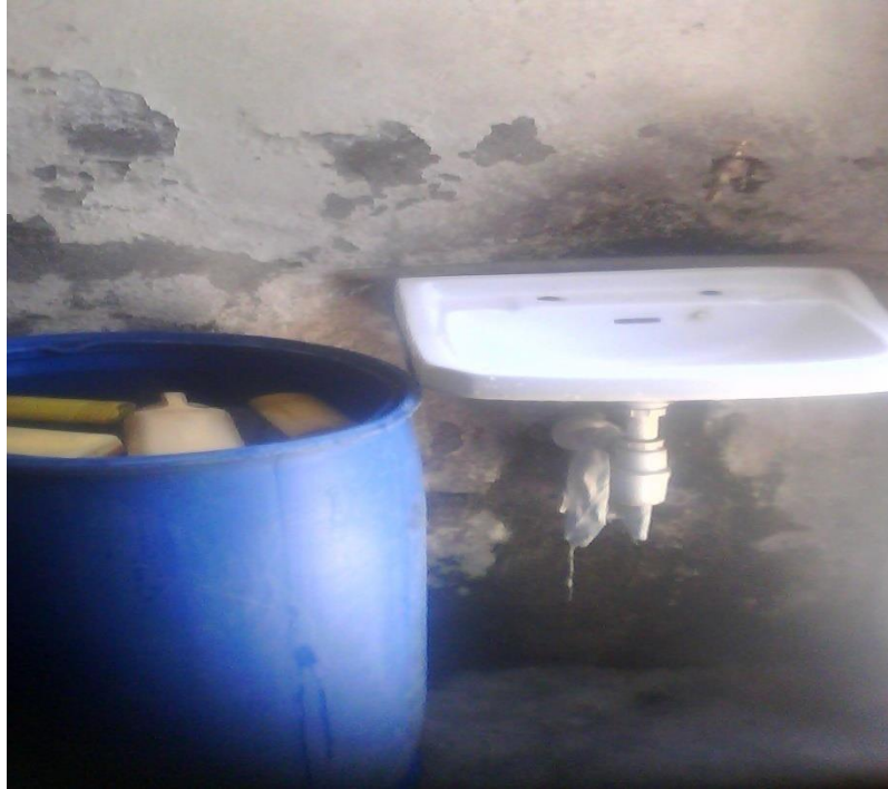
Photo graph 3: Stored water to flush latrine after use at OPD
