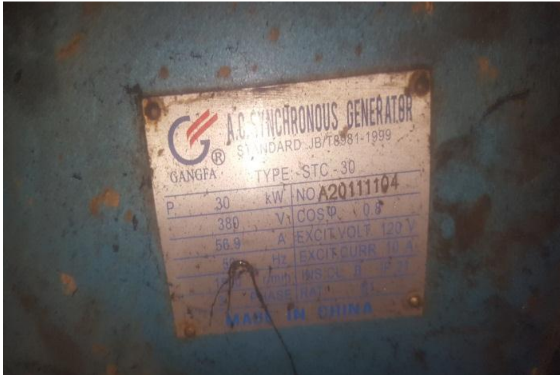
Figure 41 : synchronous generator attached to the cross flow turbine
