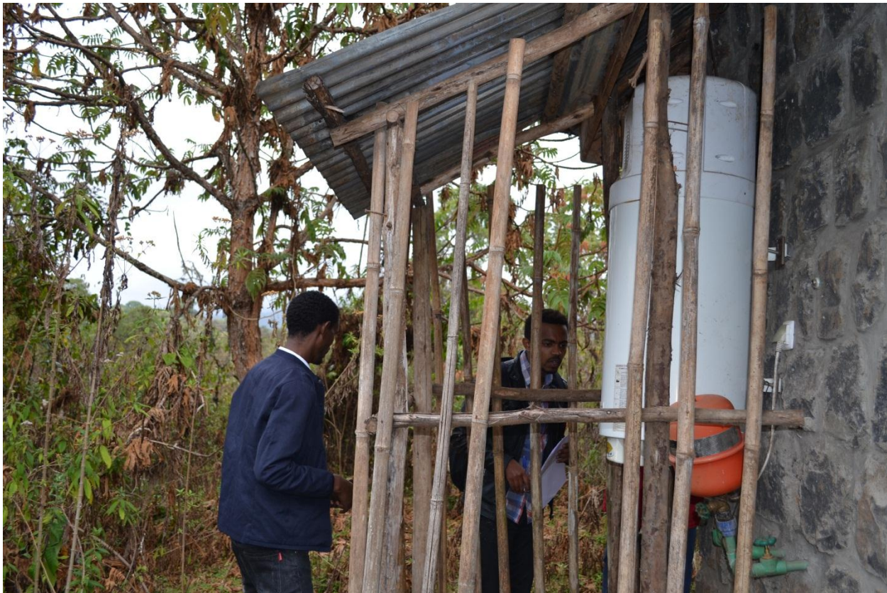
Figure 24 : a close evaluation on one of the installed heat pump system at the site
