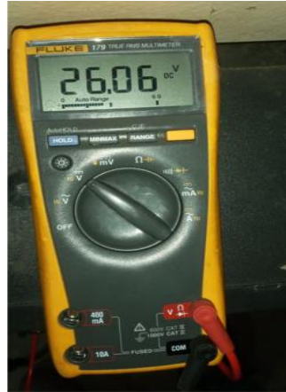
Fig.4.7. Inverter input and charge controller output voltage measurement
