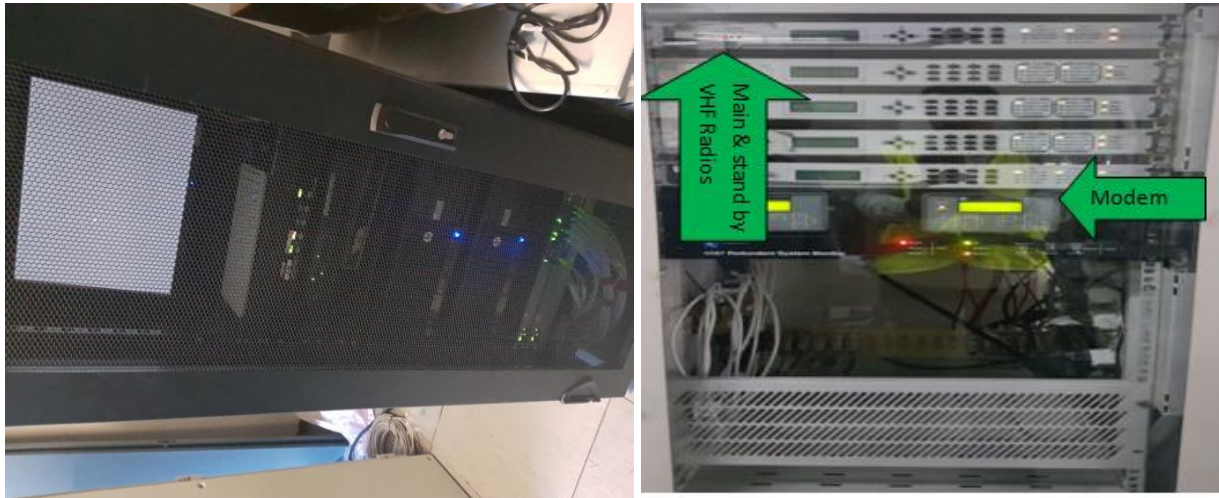
Fig.3.4. Radar and Radio loads inside a rack at ECAA
