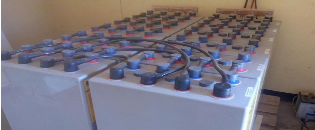
Fig.3.6. twelve newly installed OPzV valve regulated lead acid solar batteries at Arbaminch
