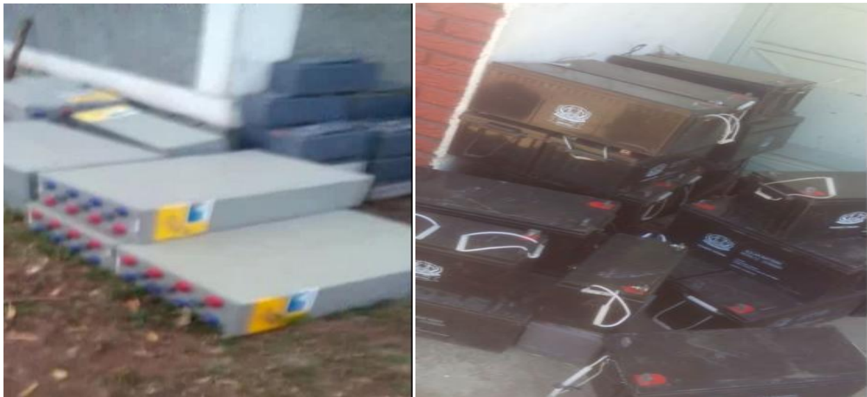
Fig.4.6. Discarded solar Batteries at Arbaminch site and at ECAA dead item store
