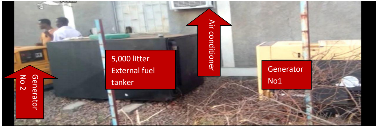
Fig.3.9. Two diesel generators at Arbaminch radio/radar station
