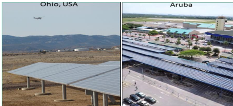
Fig.2.2. Examples of solar PV at different airports (ICAO 2017)
