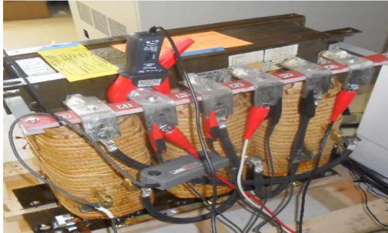
Fig.2.14. 3-Phase 208/480V delta-wye 100KVA Transformer under test (Uri and Aribisala 2013)
