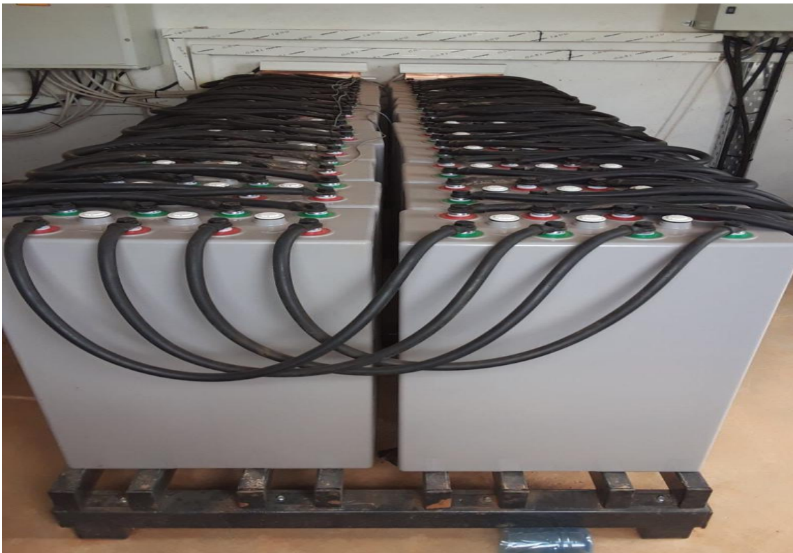
Fig.4.4. Twenty four newly installed OPZV solar batteries at Gode site
