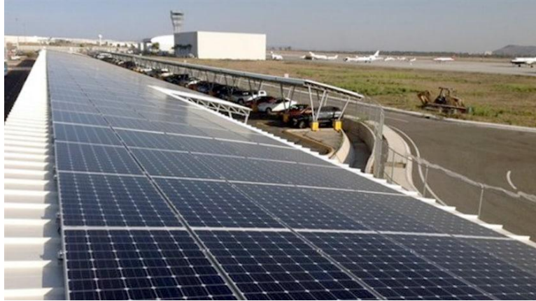
Fig.2.1. The first in African, airport Solar project, at George in South Africa (ICAO 2017)
