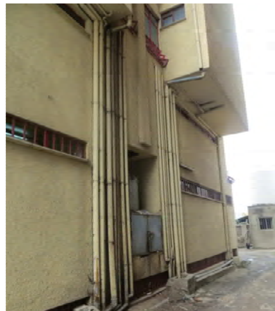
Figure 5-8 Sanitary line on external wall of ground floor by the request of the developer
