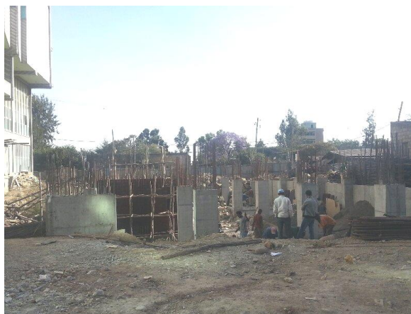
Figure 3.20 Photograph that illustrates prepared reinforcement bars prior to casting of concrete around 22 Mazonia, Addis Ababa
