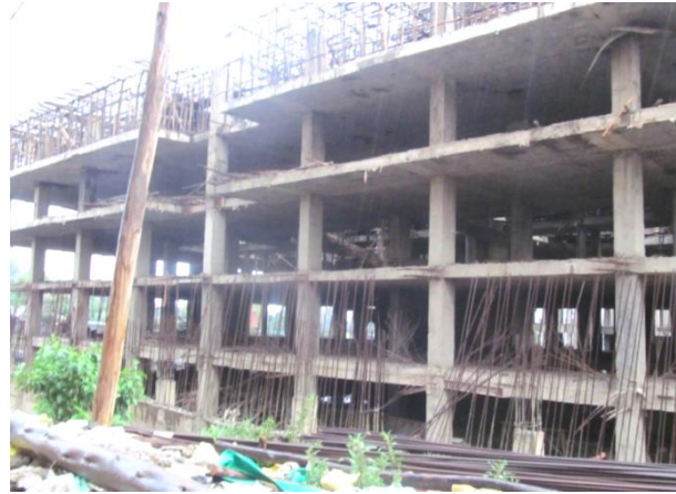
Figure 3.14 Photograph illustrating reinforcements prepared prior to casting of concrete and exposed to various environments mixed use building around Bambis area, Addis Ababa -1
