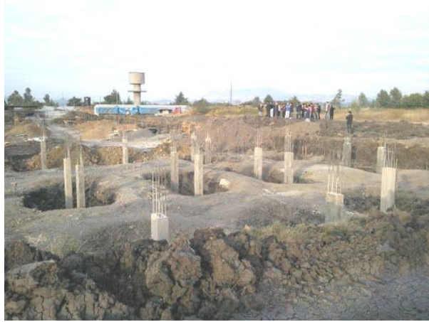
Figure 3.18 Photograph that shows prepared reinforcement bars prior to casting of concrete around Gerji area, Addis Ababa
