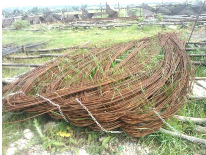
Figure 3.10 Photograph showing storage of reinforcement bar for construction of G+6 office building around Yerer, Addis Ababa - 1
