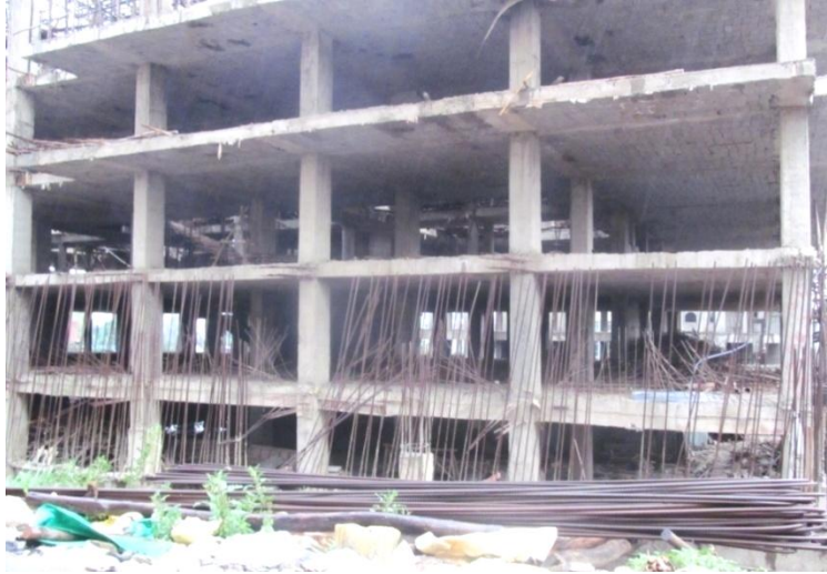
Figure 3.2 Photograph showing storage of reinforcement bar for construction of mixed use building Bambis area, Addis Ababa -1
