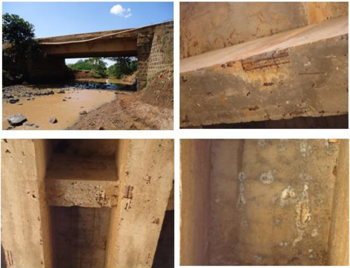
Figure 3.36 Honey comb on girder & deck slab; Cover concrete peel off; rebar exposure and water leakage on the deck slab
