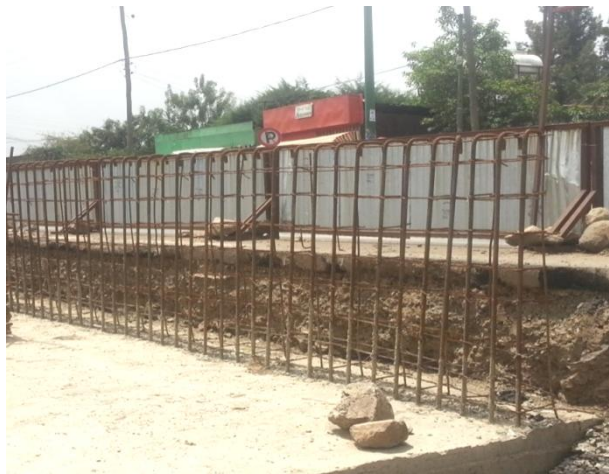
Figure 3.19 Photograph that illustrates prepared reinforcement bars prior to casting of concrete at for the new rail way project around St. Joseph Church
