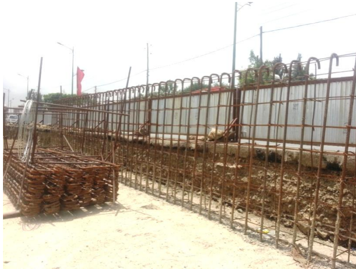
Figure 3.12 Photograph demonstrating storage of reinforcement bar for railway project around St. Joseph Church, Addis Ababa
