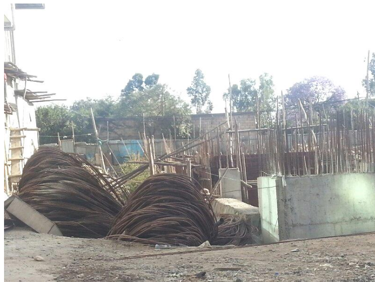
Figure 3.13 Photograph indicating storage of reinforcement bar for a mixed use building around WuhaLimat , Addis Ababa
