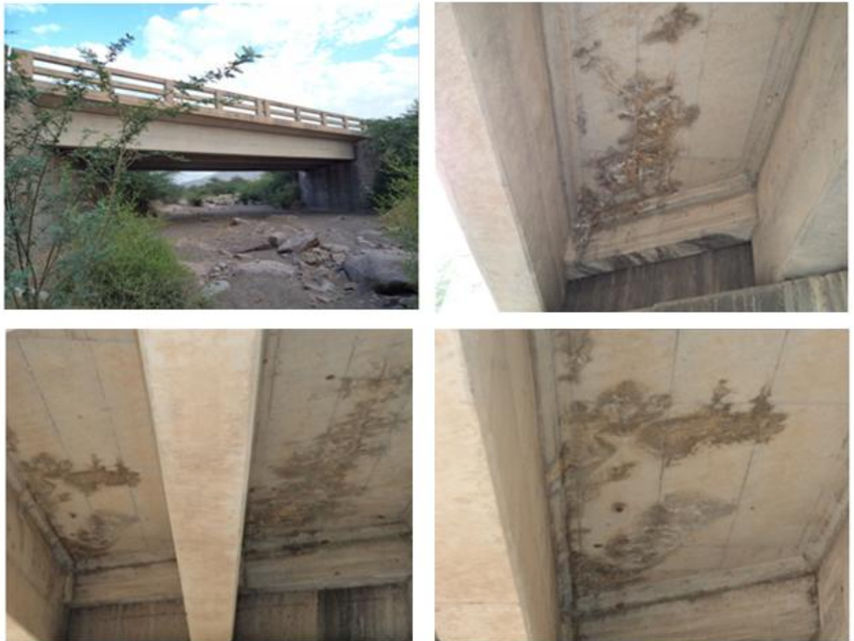
Figure 3.23 Crack and water leakage on deck slab
