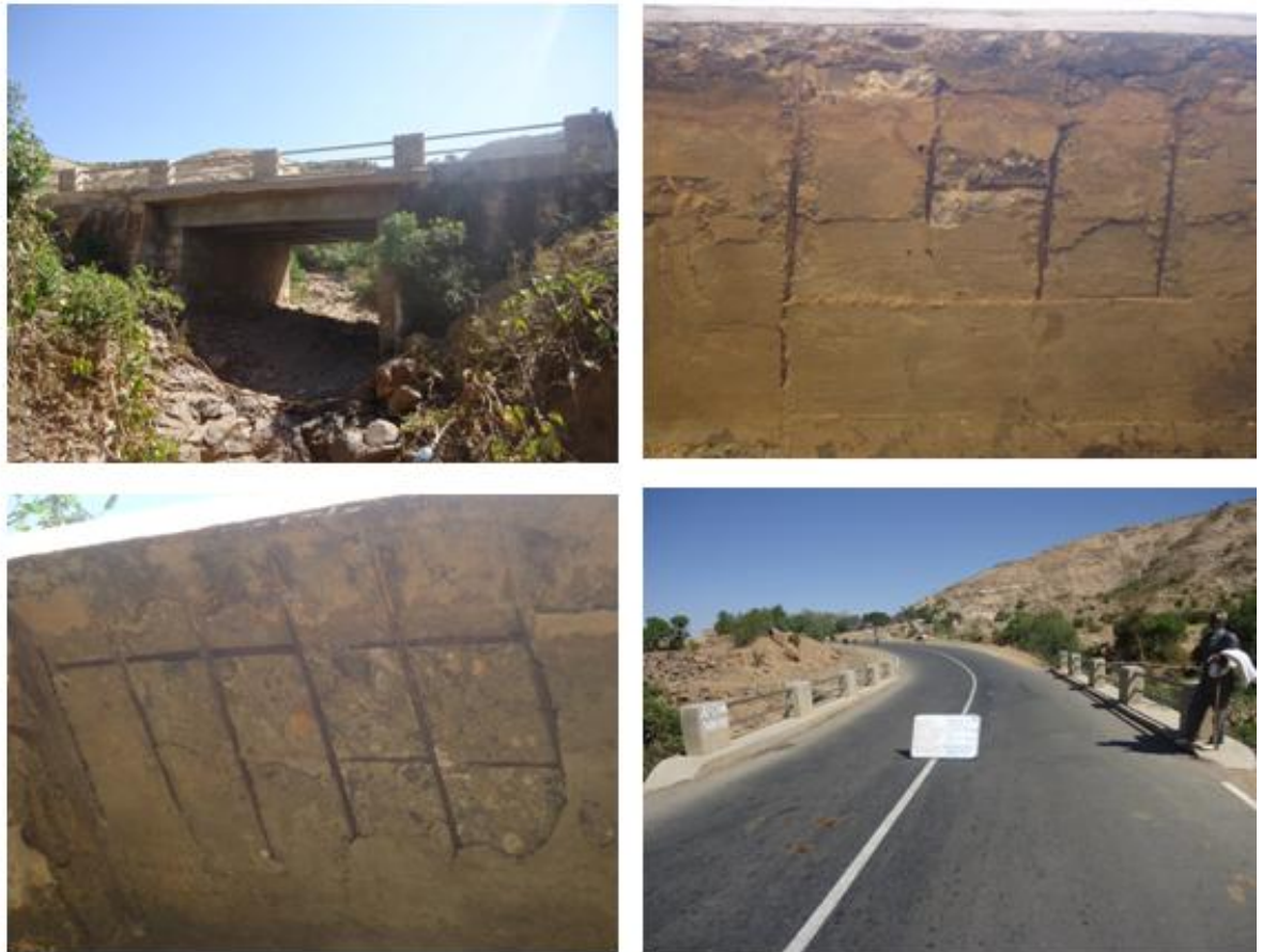
Figure 3.32 Water leakages and rebar exposure
