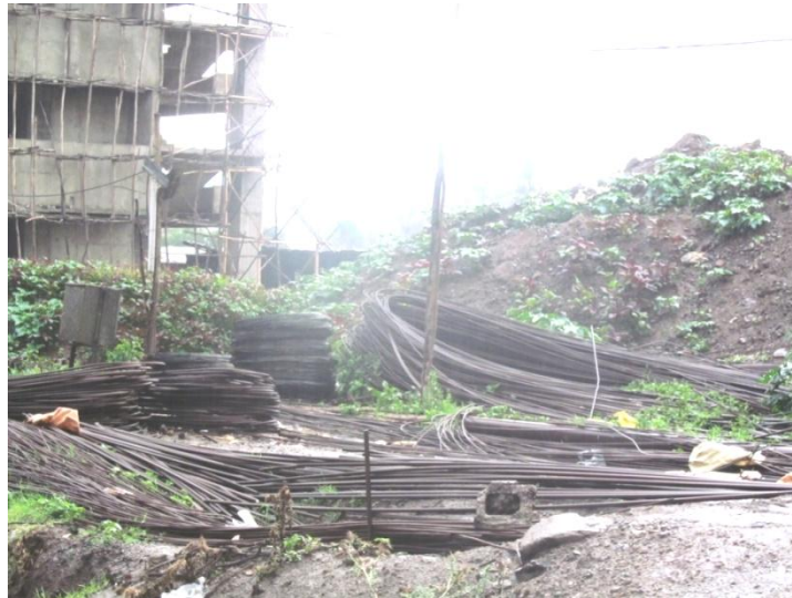
Figure 3.3 Photograph that shows accumulated reinforcement bars for construction of mixed use building Bambis area, Addis Ababa-2
