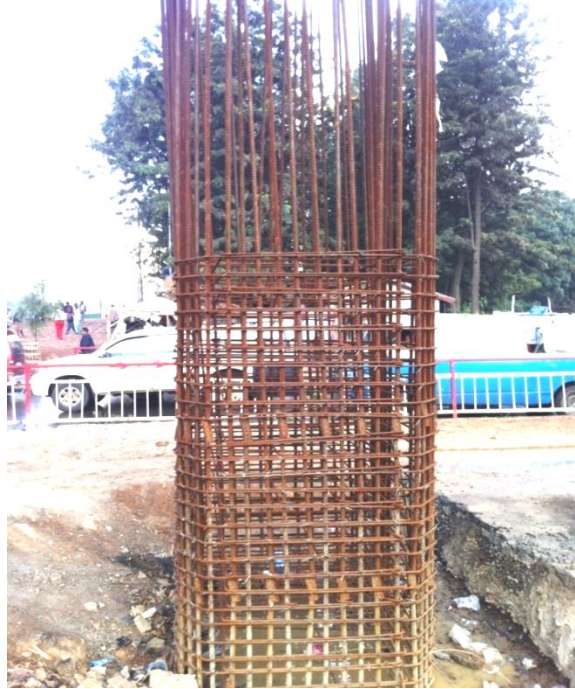
Figure 3.16 Photograph showing reinforcements prepared for footing for Railway project around Meskel square, Addis Ababa- 3
