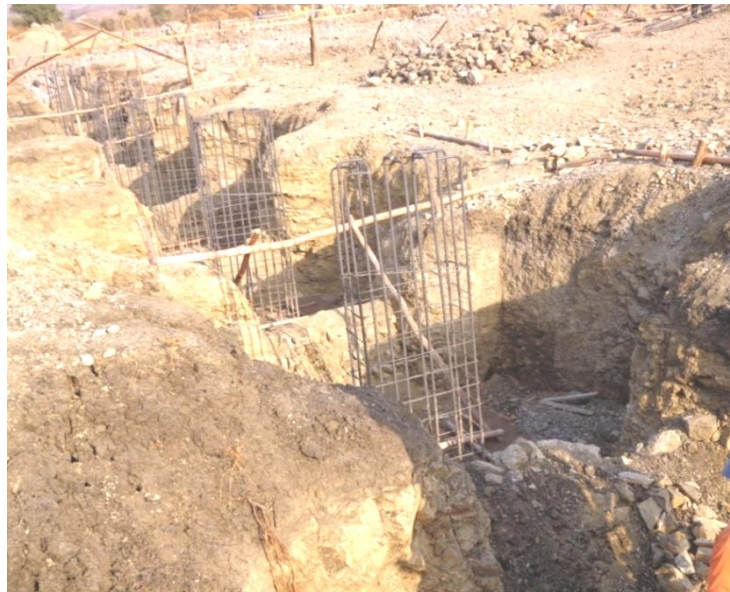
Figure 3.17 Photograph that illustrates prepared reinforcement bars prior to casting of concrete at TanaBeles sugar factory, BahirDar
