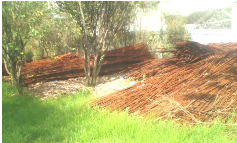
Figure 3.9 Photograph that illustrates storage of reinforcement bar for construction of G+3 parking around Kazanchis, Addis Ababa – 4
