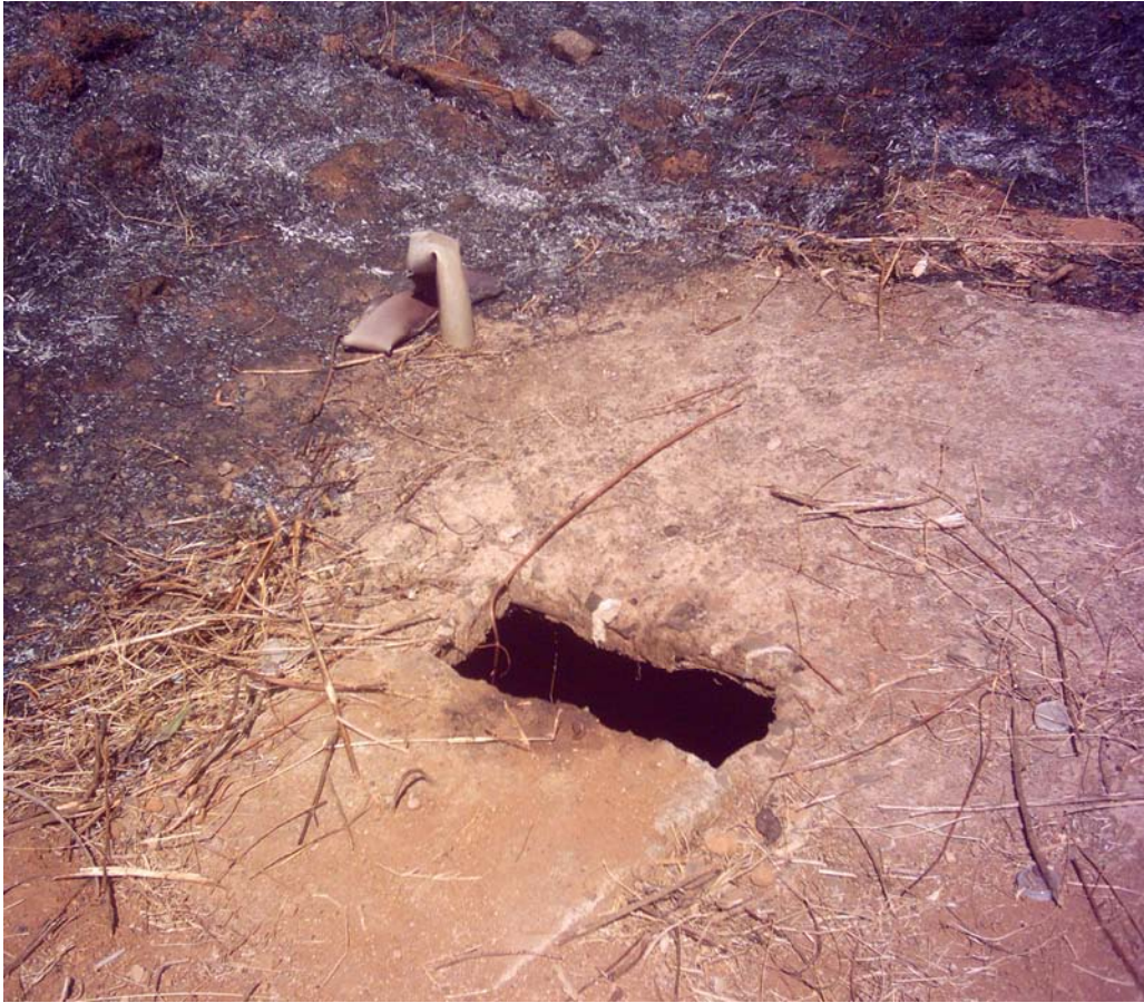
Fig 9.Placenta pit (slab made from concrete) in Dangila health center
