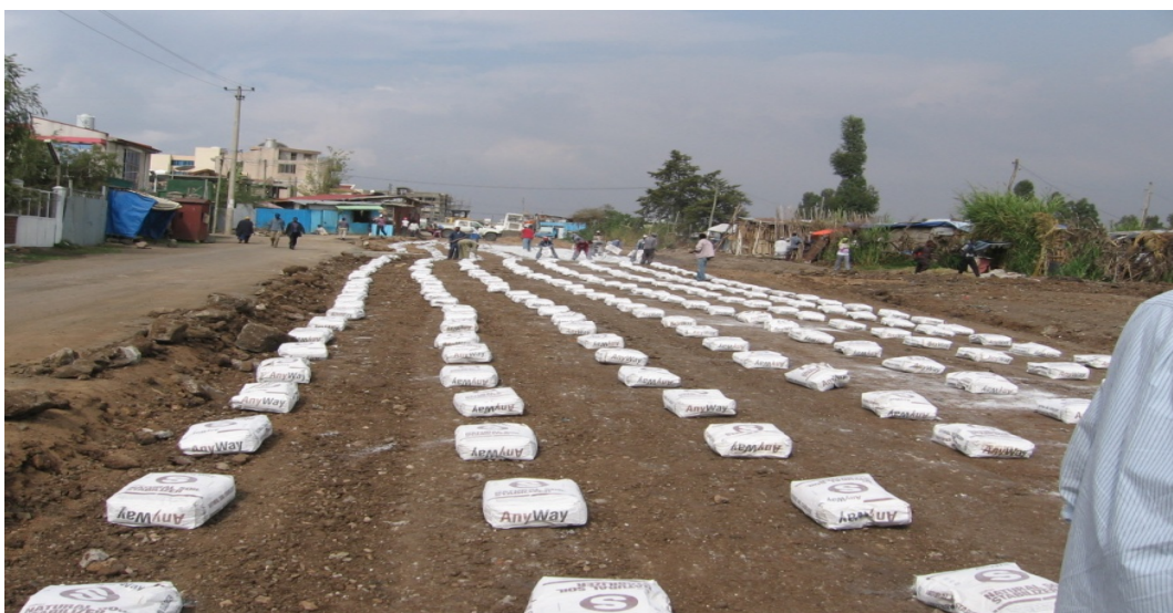
Figure 4.11: ANSS bags spread over the road section to be stabilized (Around Bole High School)
