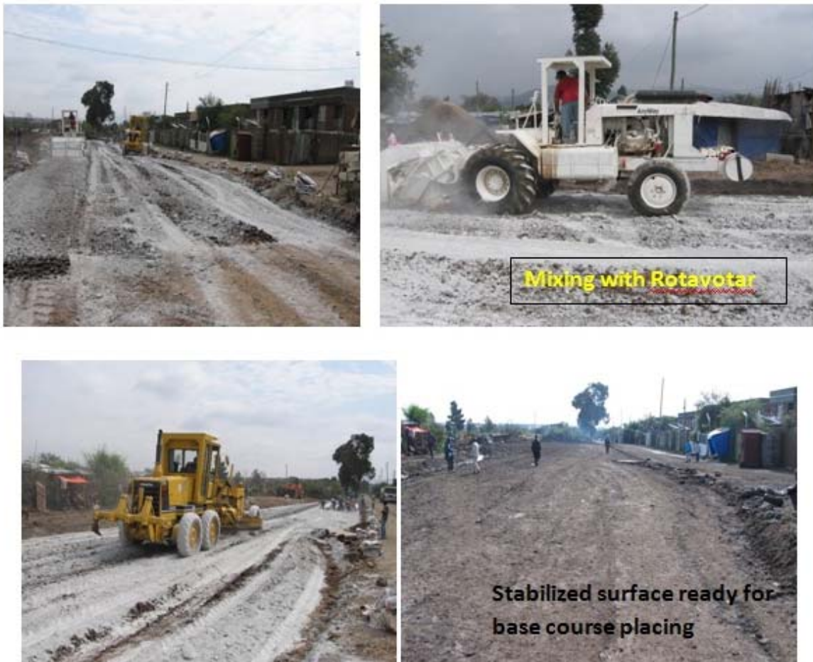
Figure 4.12: Spreading of ANSS over the surface to be stabilized and mixing with Rotovator
