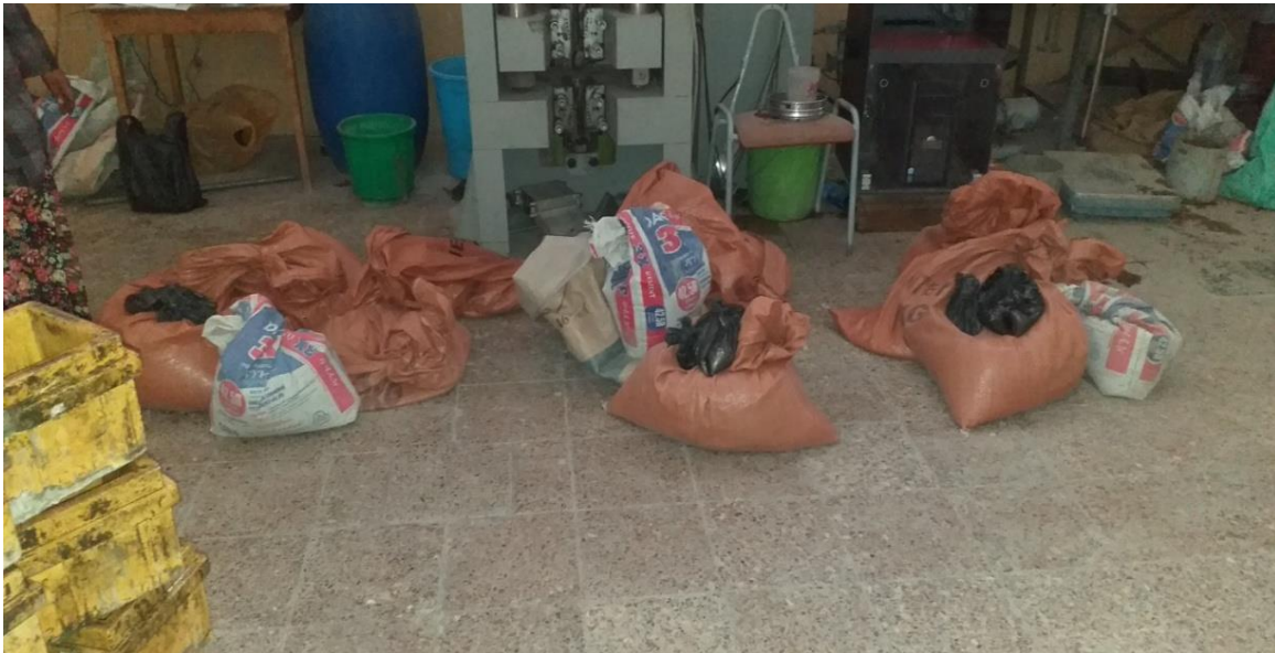
Photo 8. Concrete ingredients of different batches ready for mixing.
