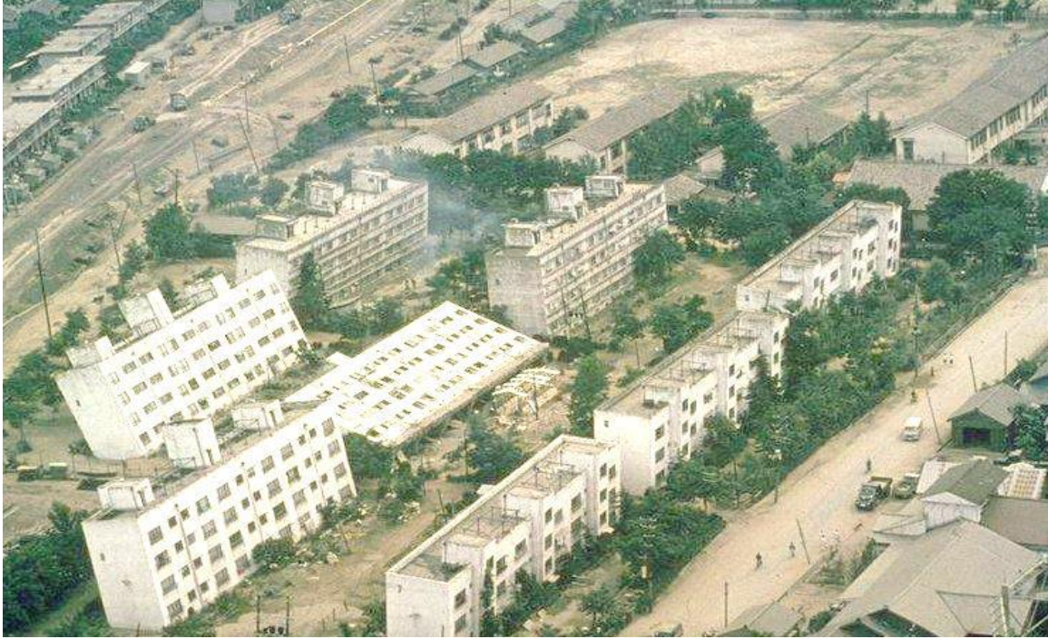
Figure 2.2 Following the 1964 Niigata earthquake, liquefaction caused bearing capacity failures in kawagishi-echo apartment buildings (courtesy of USGS)
