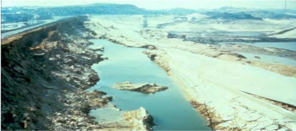
Figure 2.3 Following failure of upstream slope in the 1971 San Fernando earthquake, Lower San Fernando Dam (Courtesy of EERC, University of California)
