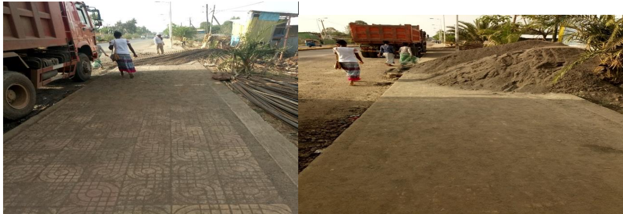
Figure 4. 3 obstacles of pedestrians due to construction materials on the sidewalk
