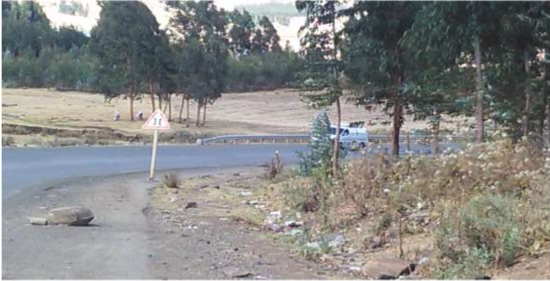
Figure-10: Ejersa Kumute Bridge and road side sight distance problem.
