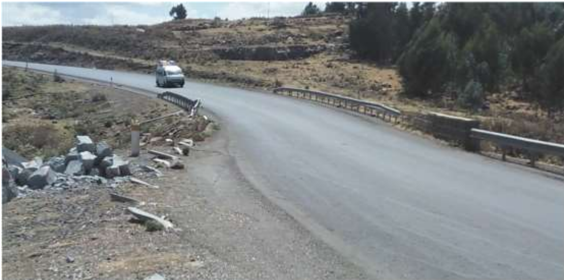
Figure-11: Ejersa kumute Bridge and guard rails under extinction by vehicles.
