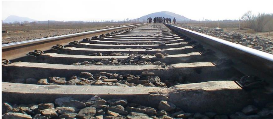
Figure 2-7 Sleeper breakage due to derailment [25].
