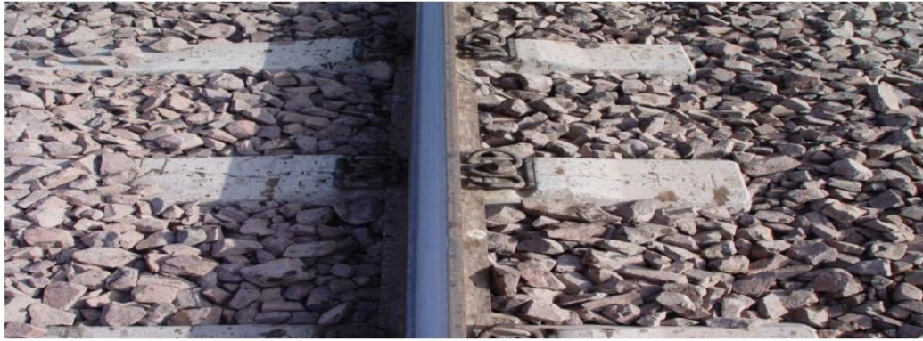
Figure 2-6 Longitudinal crack in Concrete Sleeper [25].
