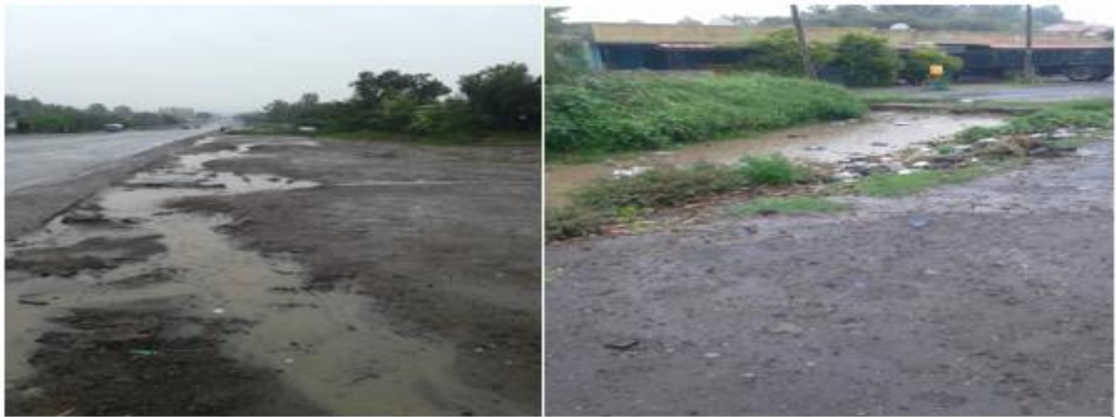
Figure 1-1 The drainage system problems on infrastructures
