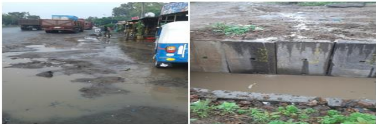
Figure 1-2 The drainage system problems on infrastructures
