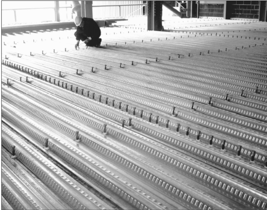
Figure 1-2: A typical example of composite construction, showing deck placing on a steel frame. Composite slabs are supported by steel beams, which normally also act compositely with the concrete slab.
