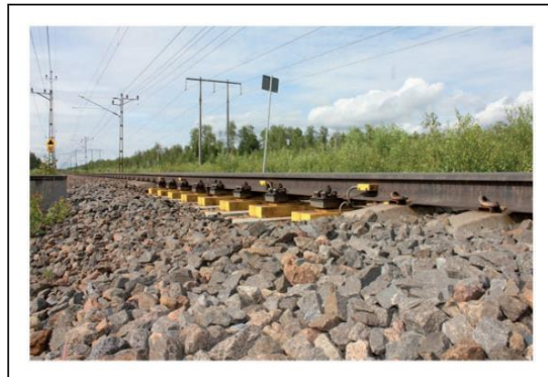
Figure 17: WDD installed along the Iron Ore Line in Sweden.[7]
