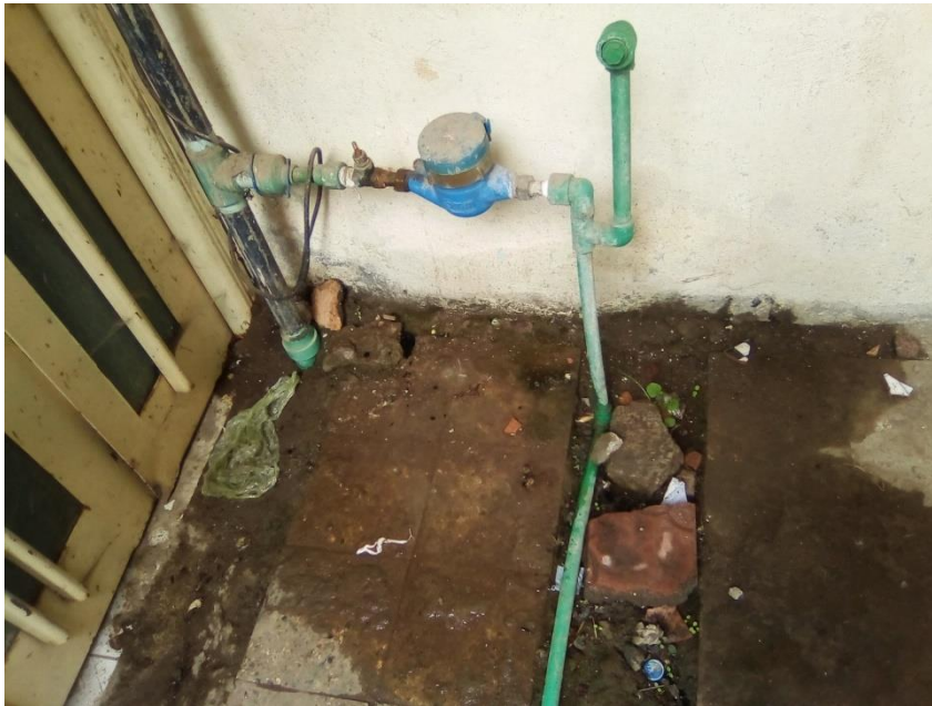
Figure 4.6 poor pipe fitting connection
