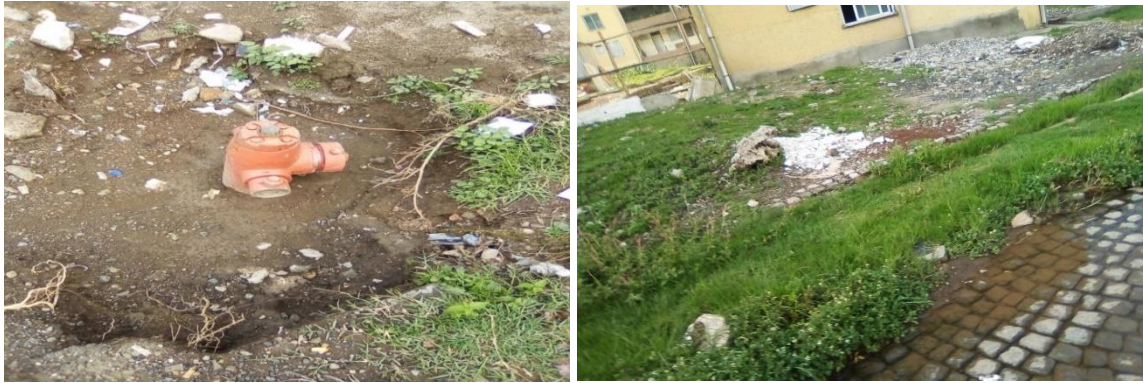
Figure 4.7 Fire hydrant without protection and unmanaged water loss
