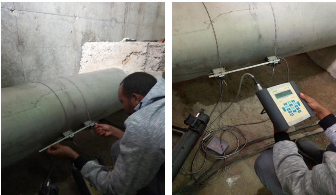
Figure 3.3 Measuring input volume of water in the system using Ultrasonic meter
