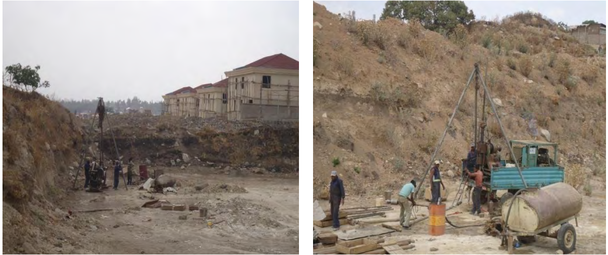
Fig. 5.11 Location in Site 8 for which SPT data was utilized in the present study
