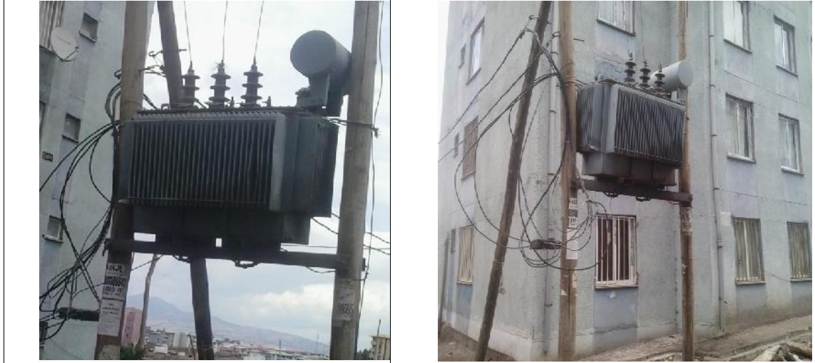
Figure 4.6: Planted transformer and fuse at Summit Condominium Housing Site (Source: photo taken by researcher from Summit Condominium Housing Site in April 06/05/2015)
