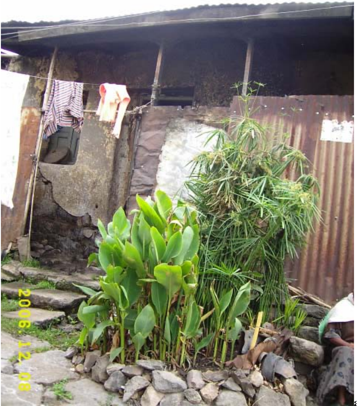
Plate14. A house lacking light and ventilation; the front part of such house (veranda) is covered with iron sheet to be used as place for cooking (kitchen).
