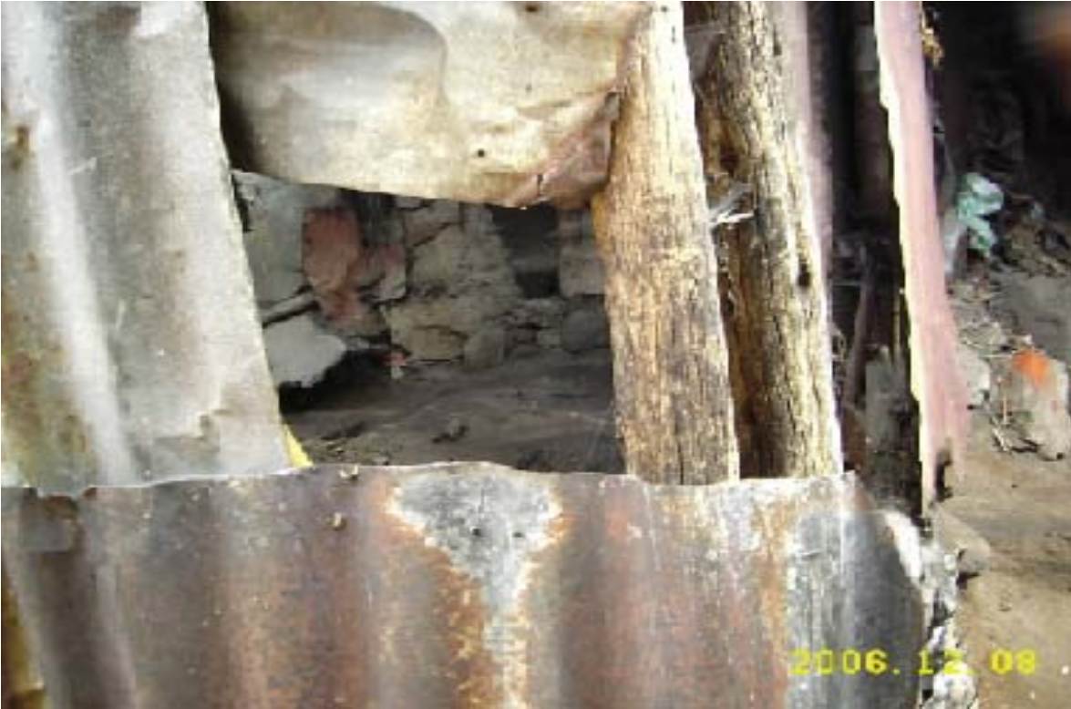
Plate 8. Toilet besides kitchen without proper walls and roof tops.
