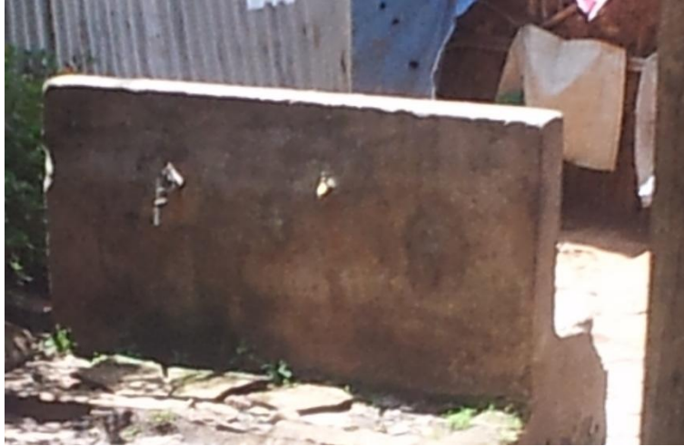
Fig 4.3. The communal pipeline, Arogew kera
