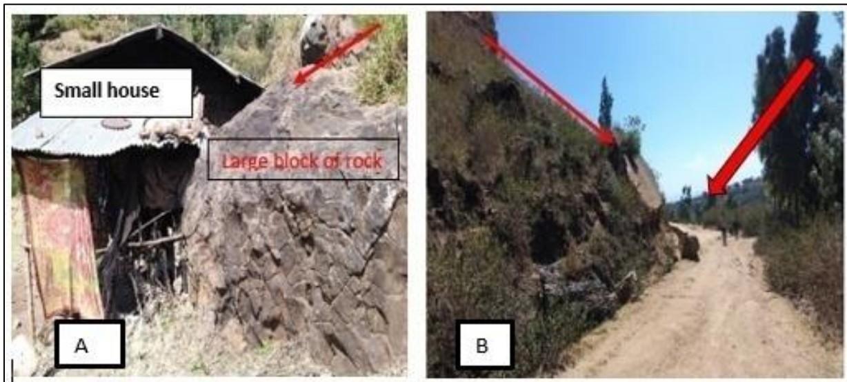
(A) Large block of rock damaged house around kundodo and (B) Rock fall damaged a gravel road from Funyan biro to Funyan-hujubo town
