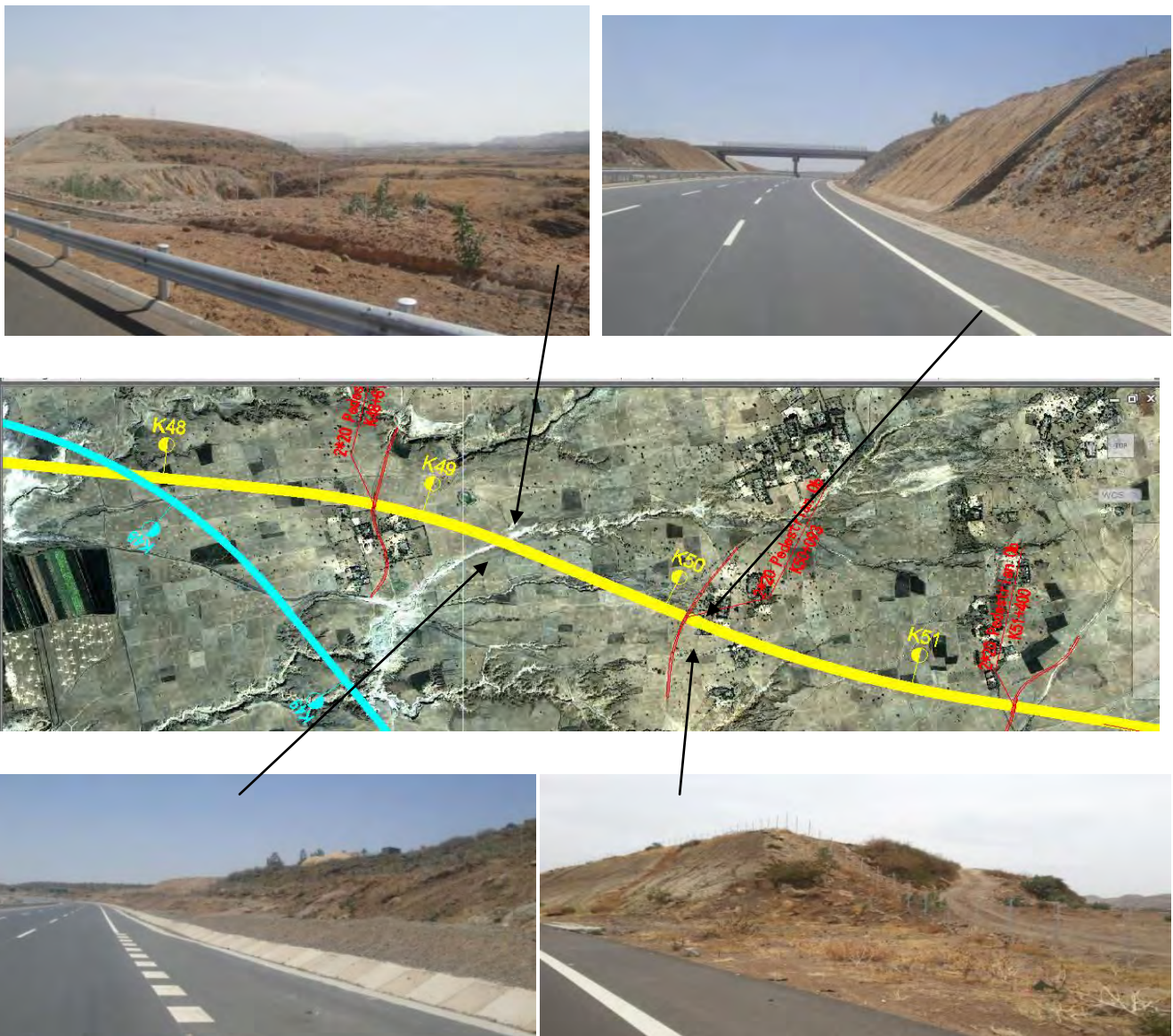
Figure 2.8a: Examples of cut batters of the Express still not stabilized.(Route of Express way highlighted yellow) 1
