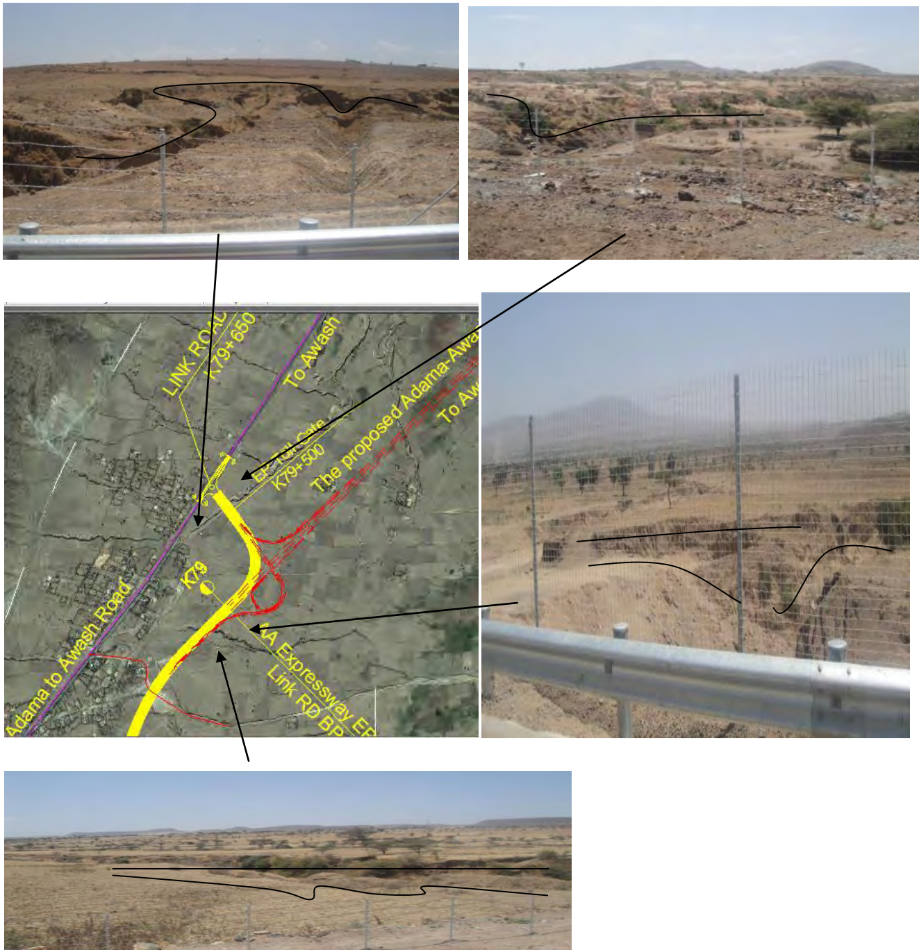
Figure2.5b; Severely eroded gullies near the Express way. (Route of Express way highlighted yellow) 1
