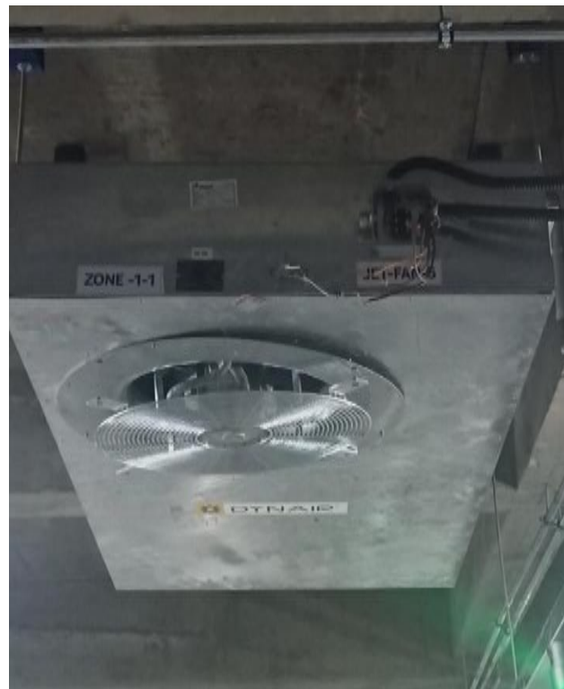
Figure 15: Jet Fans (Centrifugal Fans)
