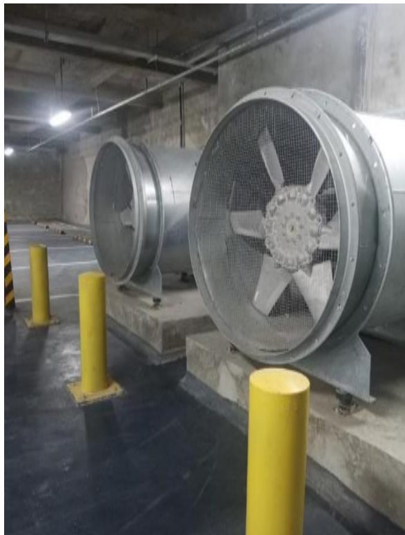
Figure 14: Supply Fans (Axial Fans)
