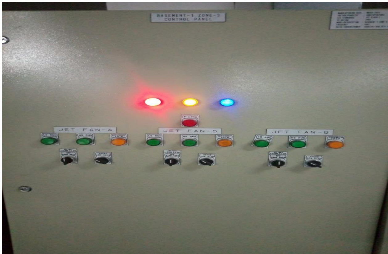
Figure 18: Meskel Square Ventilation Fans Control Panel
