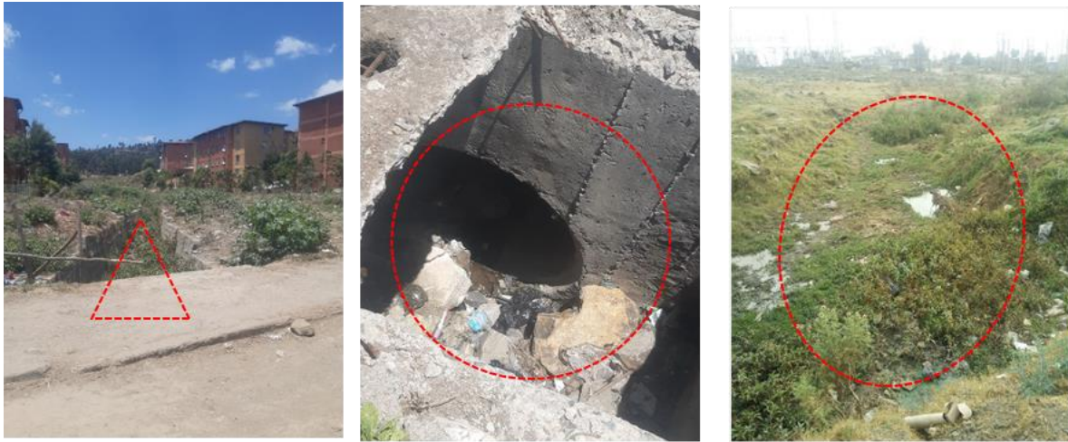
Figure 4:17: Drainage conditions at Ayat Tafo condominium Source: Photo taken by the researcher, 2025
