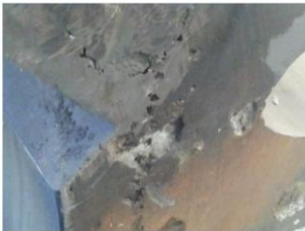
(e) Surface crack
