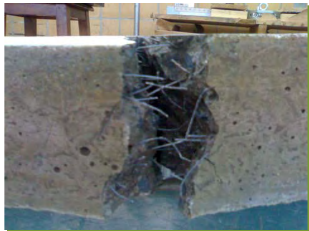
Fig. A.J-48 A Beam Failed in Flexure
