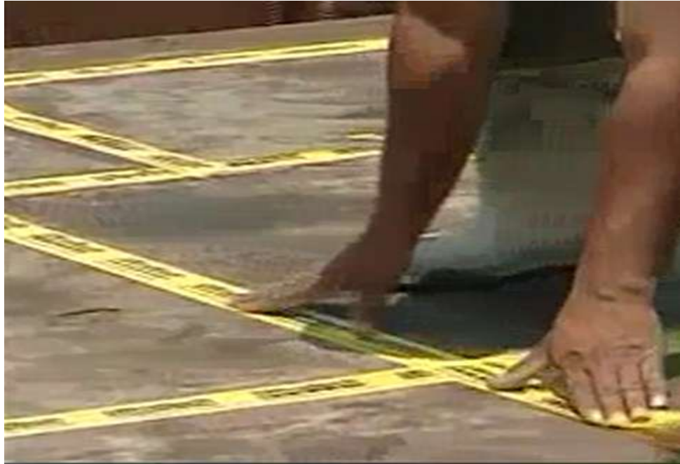
Figure 2.2 Sealing gaps between form sheets with mastic tape to prevent slurry leakage (Ultratech Services, 2014)
