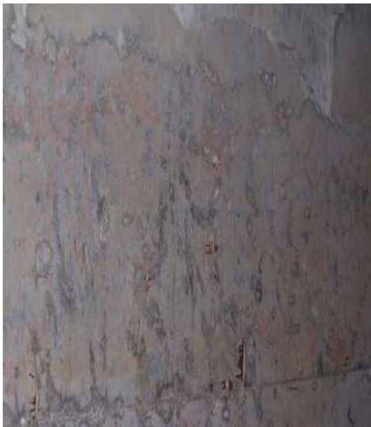
(c) Plywood Grains Stuck on Concrete Surface
