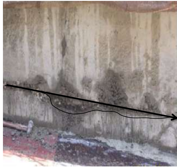
(b) Poor Construction Joint/Offsets in Concrete
