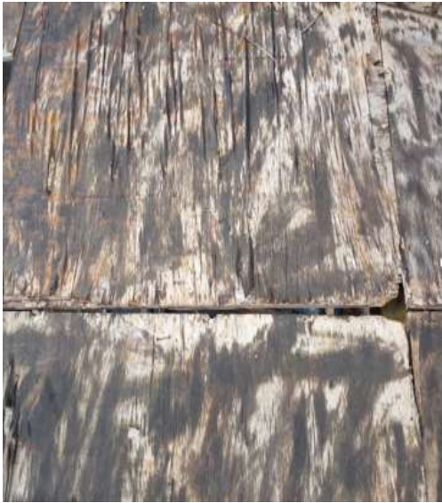
(a) Inadequate application of form oil
