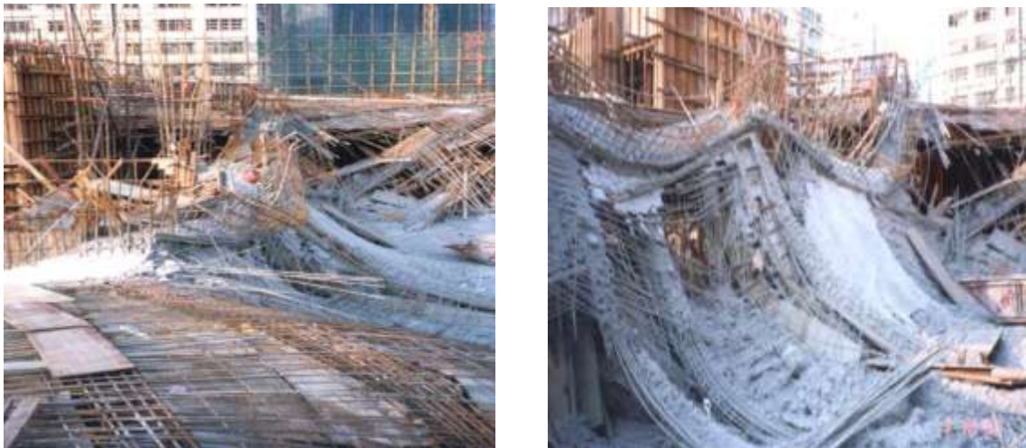
Figure 2.14 Formwork Collapse Cases - Industrial Building in Kwai Fook Rord (Chung, 1995)
