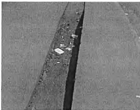
Figure 4.6 Picture showing Un maintained roads
