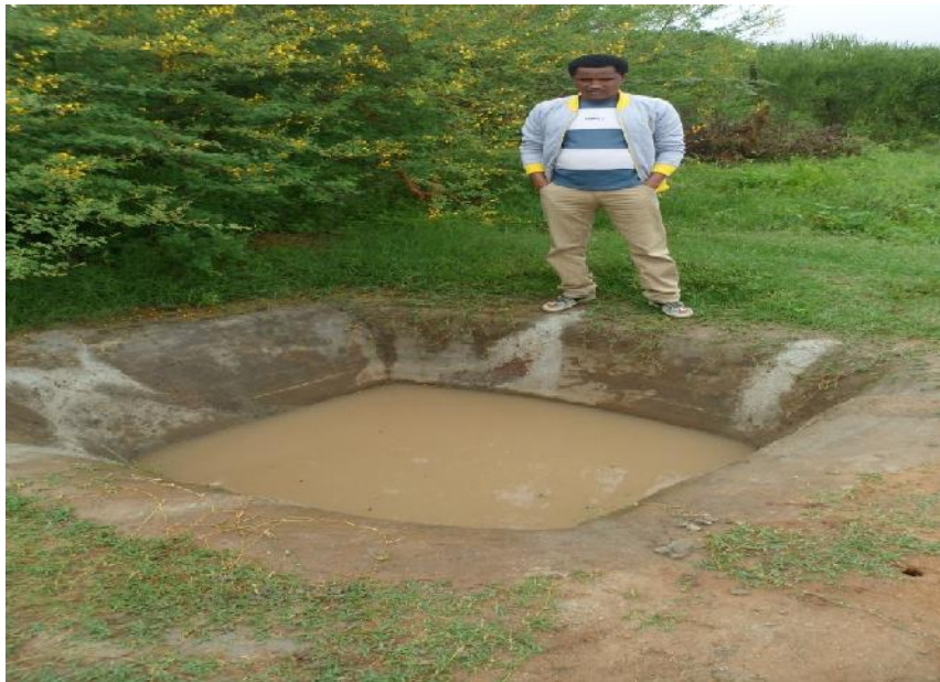
Fig 4.10 Farmers used to clean concrete tanks till two to three years after construction (photo by author)
