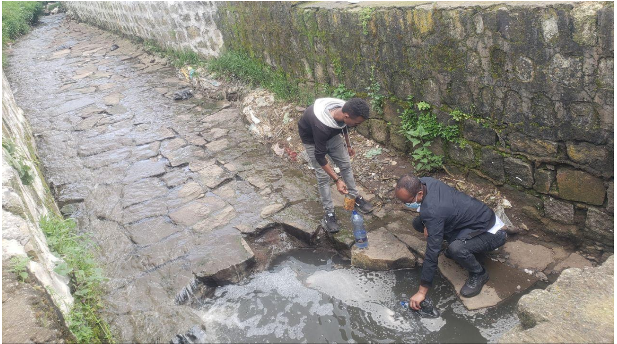
Figure 9: The status of residential sewerage system near to Ethiopian Science academy, 2022
