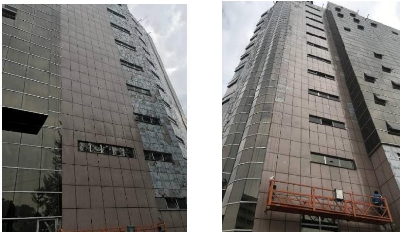
Figure 4.13 Defects seen on children and youth theatre building
