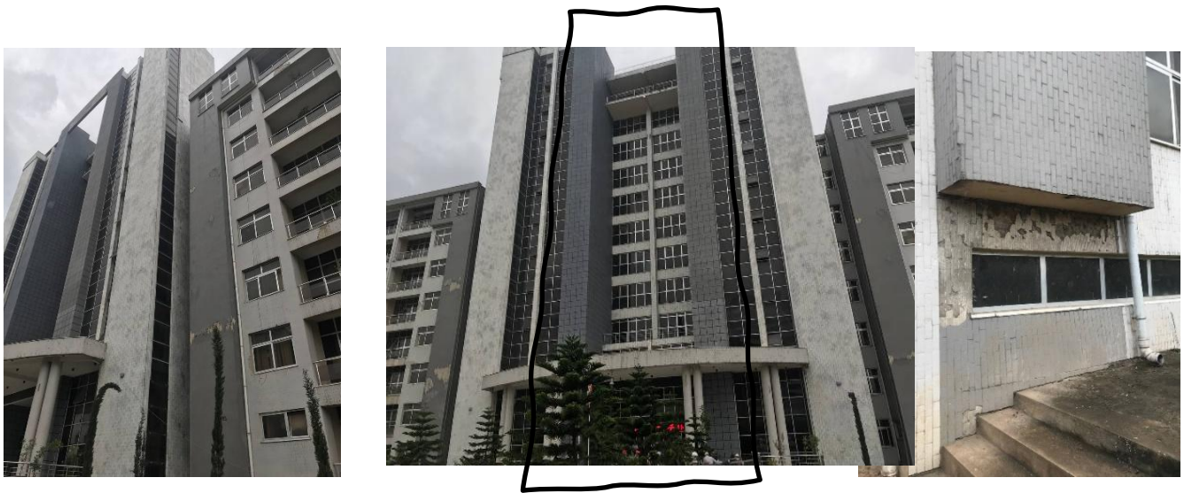
Figure 4.12 Defects seen on Bole sub city administration building (B+ G+12)
