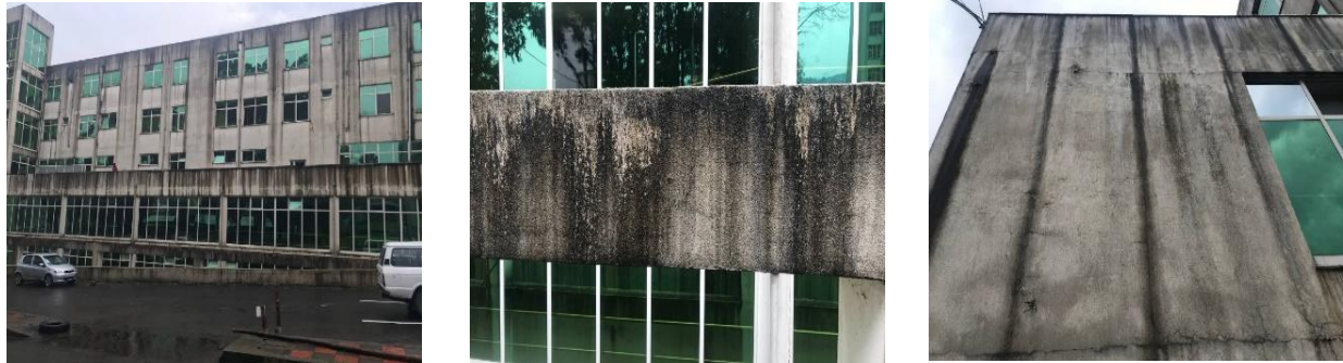
Figure Error! No text of specified style in document..13 Defects seen on exterior finishes of St. Peter hospital (MOH)
