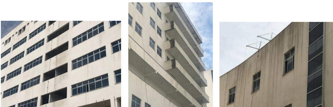
Figure Error! No text of specified style in document..12 Defects seen on exterior finishes of St Paul millennium hospital (MOH)
