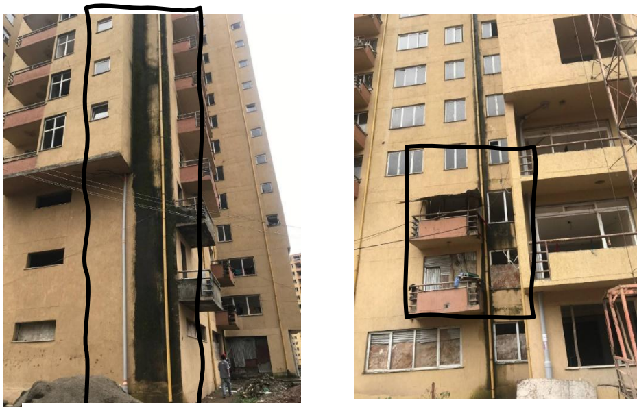
Figure 4.15 Defects seen on 40/60 condominium housing project
