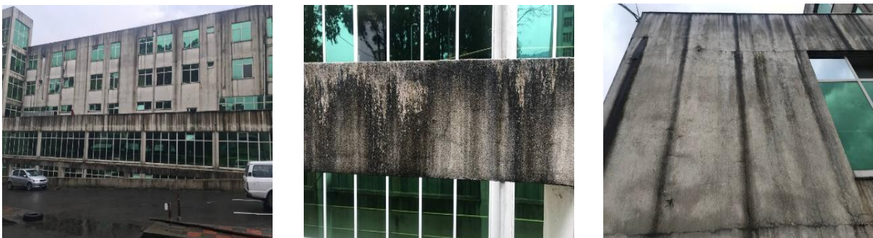
Figure 4.17 Defects seen on exterior finishes of St Peter hospital (MOH)
