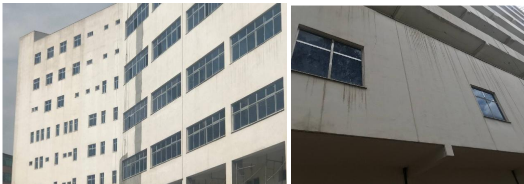
Figure 4.8 St Paul hospital, cardiac building
