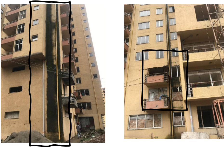
Figure Error! No text of specified style in document..11 Defects seen
