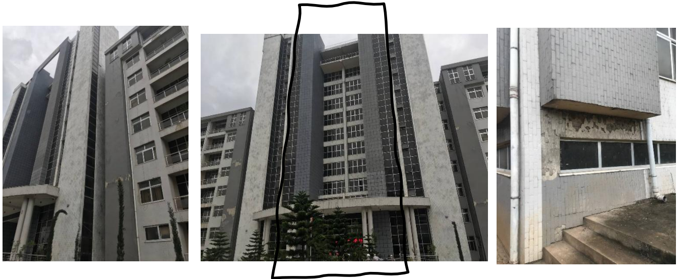
Figure Error! No text of specified style in document..8 Defects seen on Bole sub city administration building (B+ G+12)
