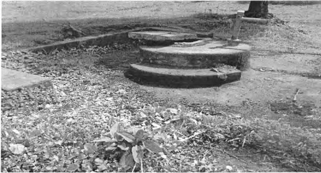
FIGURE-2: Non-functional scheme (found in Gari Kebele, Dinsa Shone village) because of lack of maintenance.
