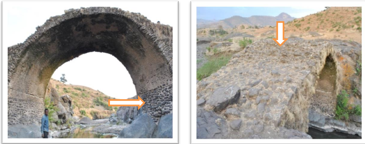
Figure 3.32. The base of the Bridge eroded by the rainy flood (left figure), and its deteriorated surface (right figure) (Photo by Kedir 2018)
