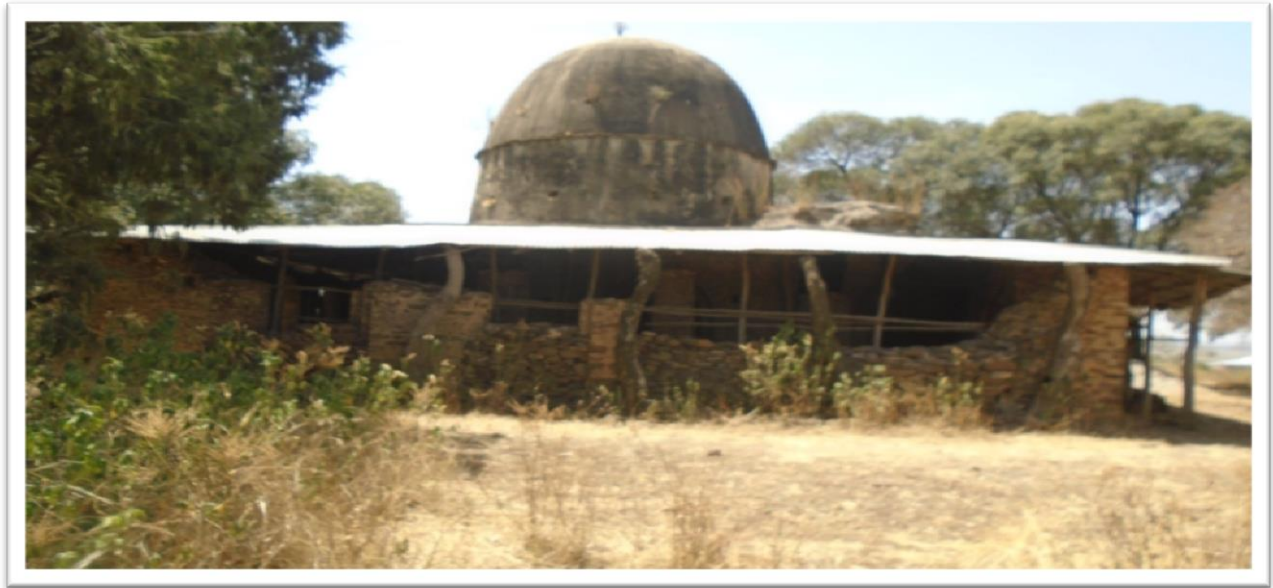
Figure 3.54 Northern face of Bahri Ginb, destroyed but repaired with stones without keeping the authenticity of the original Building (Photo by Kedir 2018)
