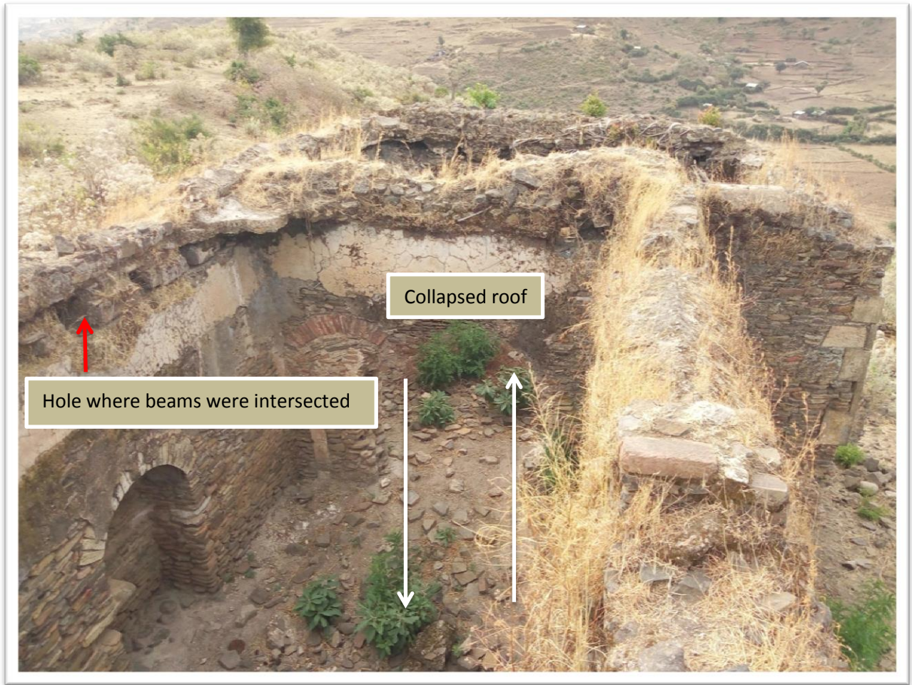
Figure 3.40 Aerial view of the Building, showing how much it is deteriorated (Photo by Kedir 2018)
