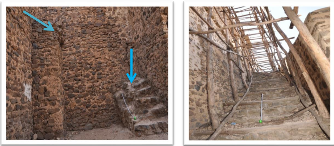
Figure 3.3. A destructed staircase inside the palace leading to the upper floor (the left figure); the outside stair case (the right figure) (Photo by Kedir 2018)
