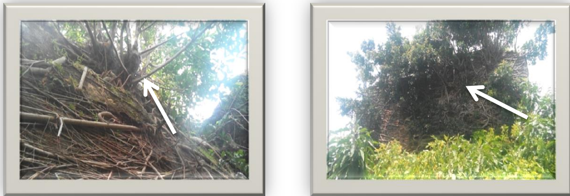
Figure 3.39 Trees grown on the building: at inside (left figure), and at outside, the eastern face (right figure) (Photo by Kedir 2017)
