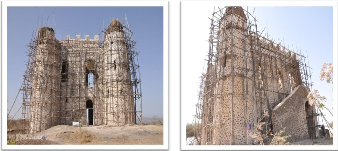
Figure 3.17. Guzara Palace on Conservation: the northern face (left figure), and the western face (the right figure) (Photo by Kedir 2018)
