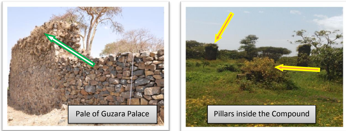
Figure 4.16. Mortar Deterioration, decay and damage of the Guzara Palace due to Biological Causes (Photo by Kedir 2017/2018)
