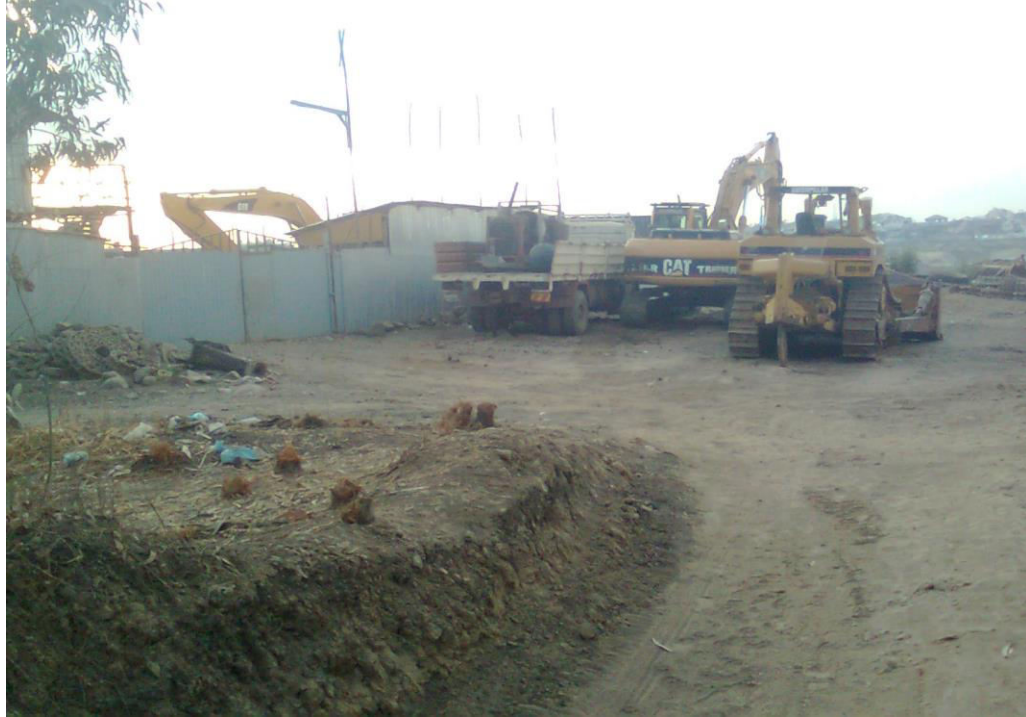
Picture 03-Crusher plant site and the heavy trucks (photo by the author-03/02/2014)
