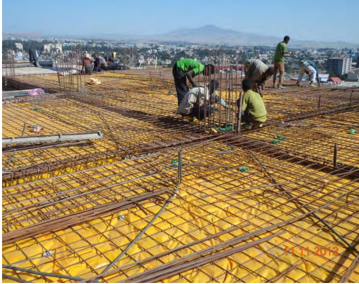
Fig. 2.18 Slab formwork construction systems for office building around Megegnsgnai in Addis Ababa
