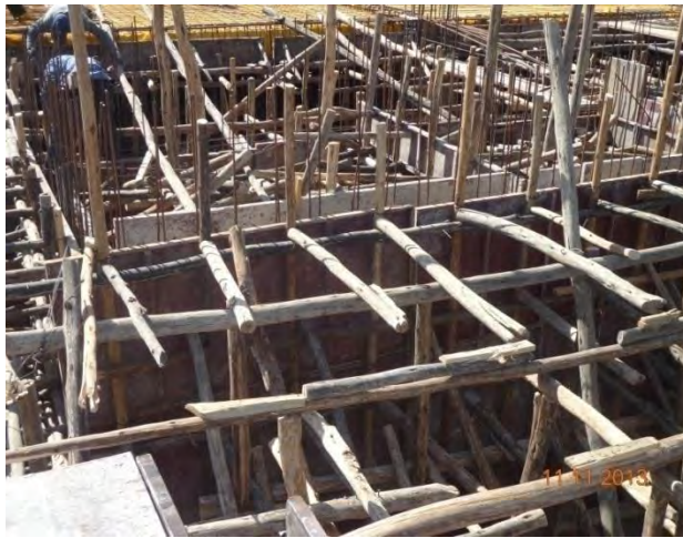
Fig. 2.17 Shear wall formwork construction systems in Addis Ababa around Megegnagnai for office building
