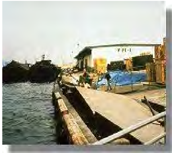
Retaining wall damage and lateral spreading, Kobe 1995
