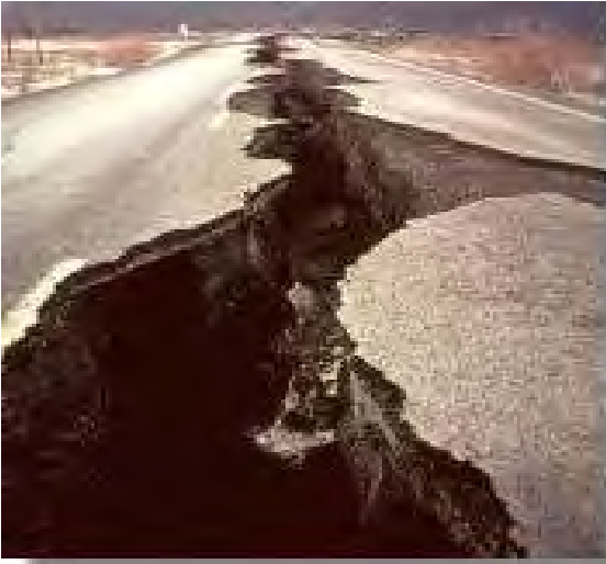
Cracked highway, Alaska, USA 1964
