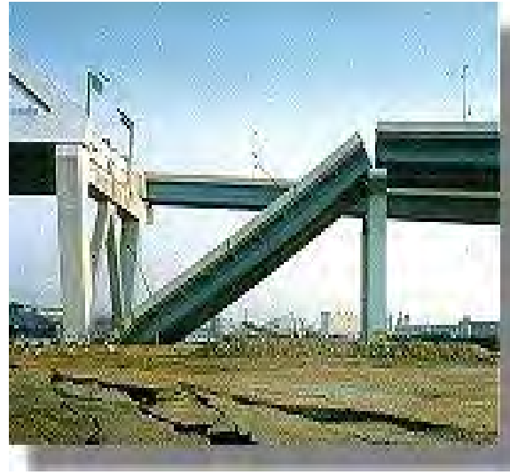
Collapsed bridge, Kobe, Japan, 1995
