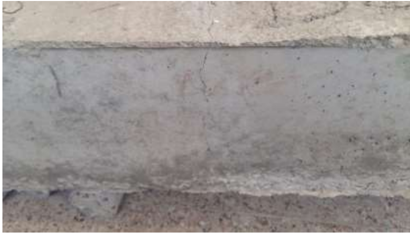
Figure 5.1 : Damage on B1M
