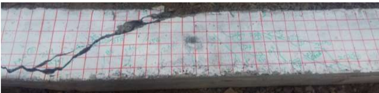
Figure 5.11 : B2C80 after failure
