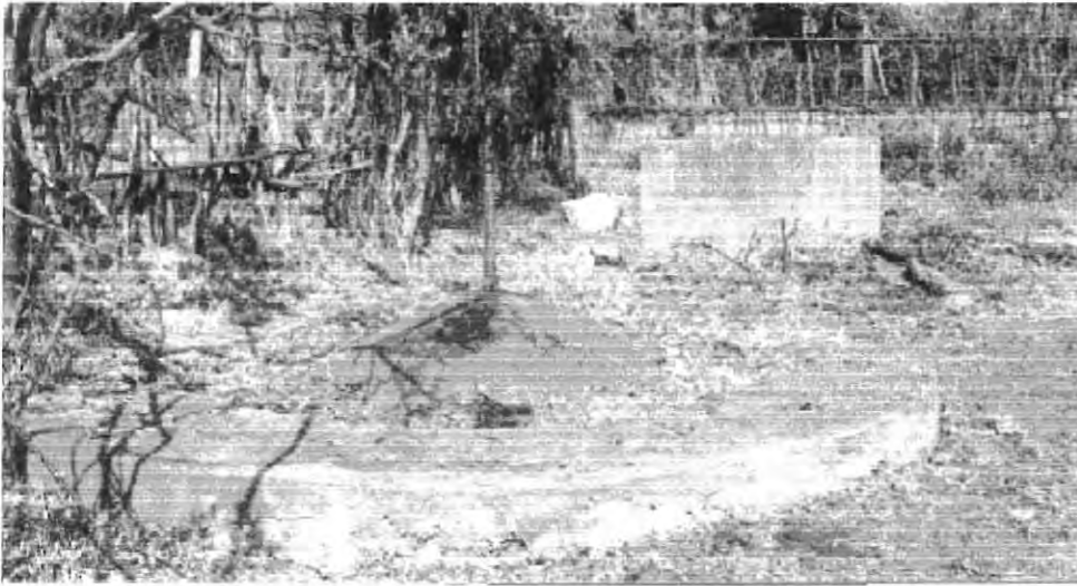
Figure 5.1 Status of Biogas Digester Found at Inewonta (Yetnora) Village
