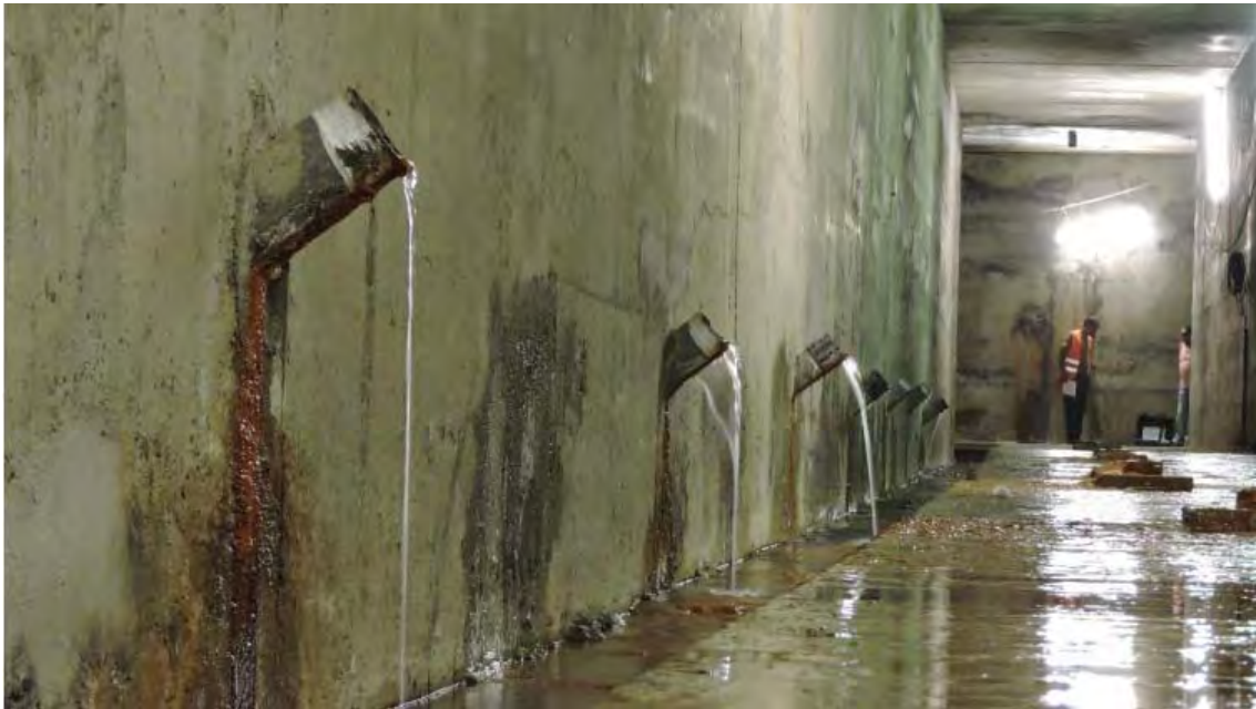
FIGURE 3. 3: Seepage from gallery at 660 m.a.s.l
