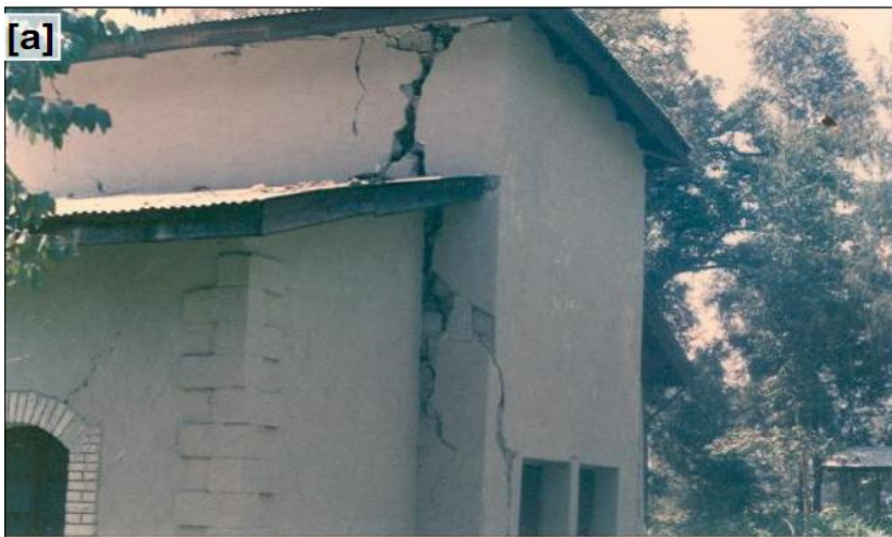
Figure 2.1 Damage to Wetera Abbo Church in Wondo Genet during the 1983 earthquake [3]
