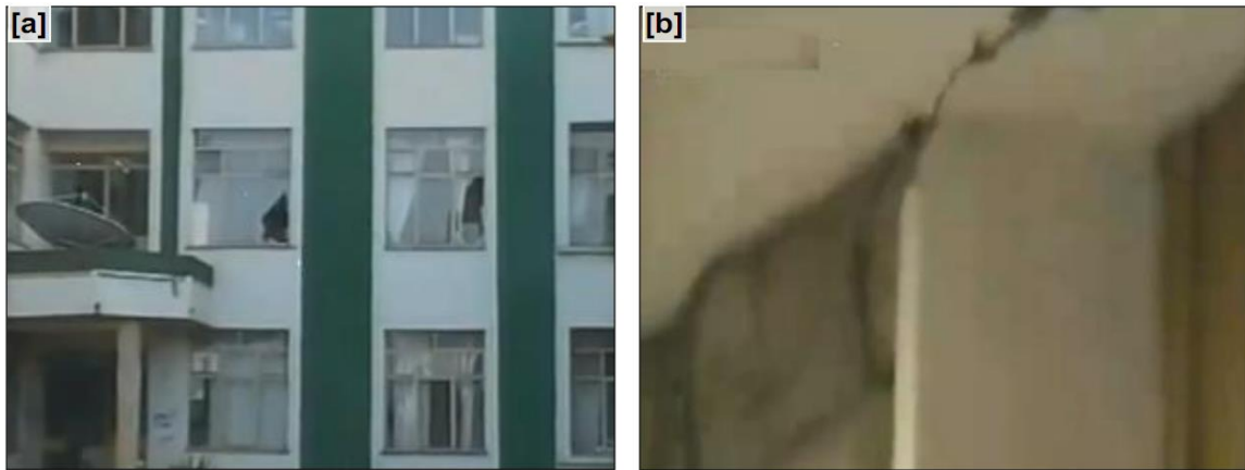
Figure 2.2 Structural damage in December 2010 Hossana earthquake.
