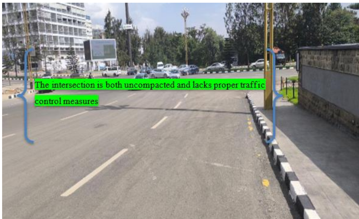
Figure 16 Uncompacted and lacks proper traffic control measures
