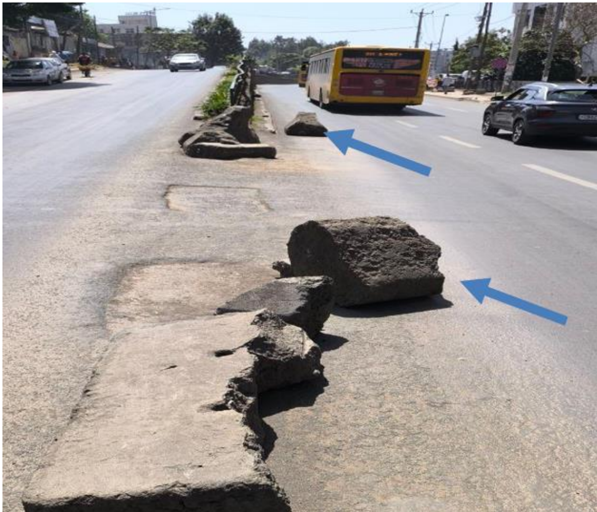
Figure 7 Obstructing the vehicle path.
