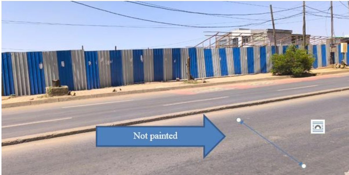
Figure 5 Absence of Correct type of longitudinal line markings
