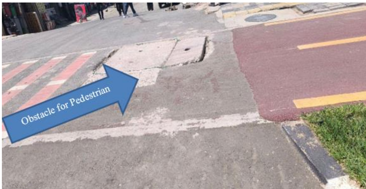
Figure 20 Pedestrian safety and cycle lane discontinuity
