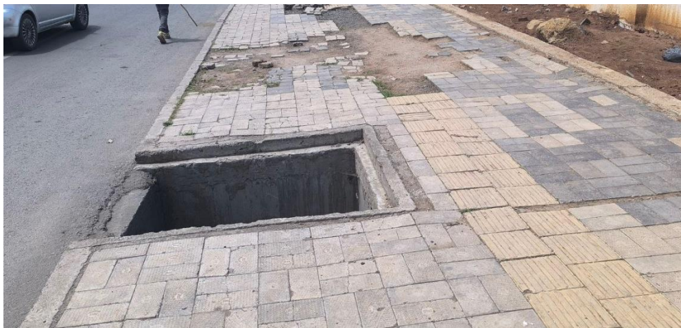
Figure 14 Extremely dangerous man hole
