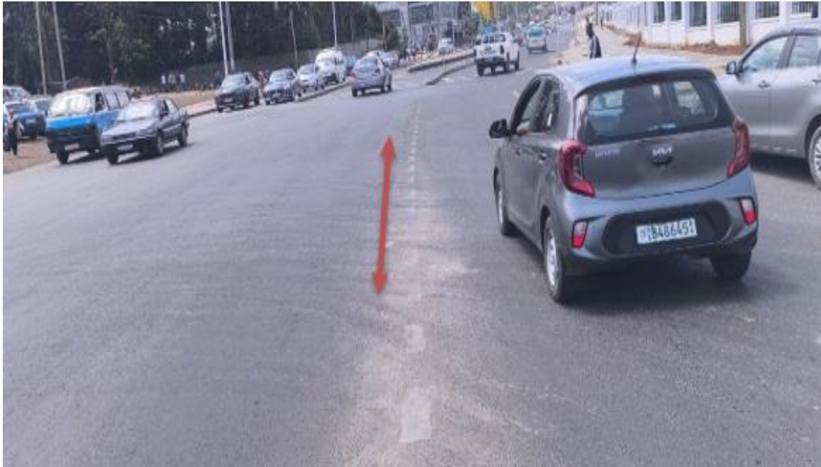
Figure 15 Missing or faded median and lane division lines
