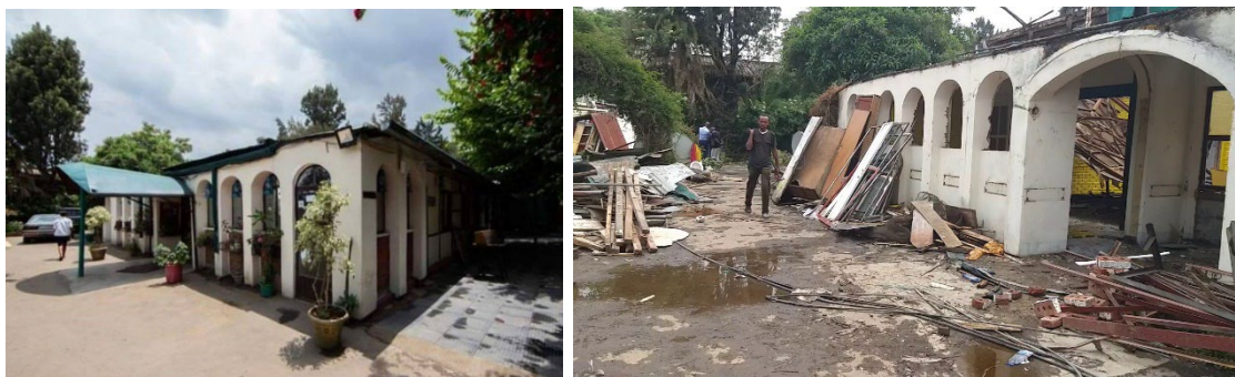
Figure 4-4: Before [Left] and After [Right] Demolition Photo of Buffet De La Gare Source: Left Photo – Video of the demolition posted by Piassa Tube on 18 January 2019, Right - https://addisfortune.news/bulldozed/
