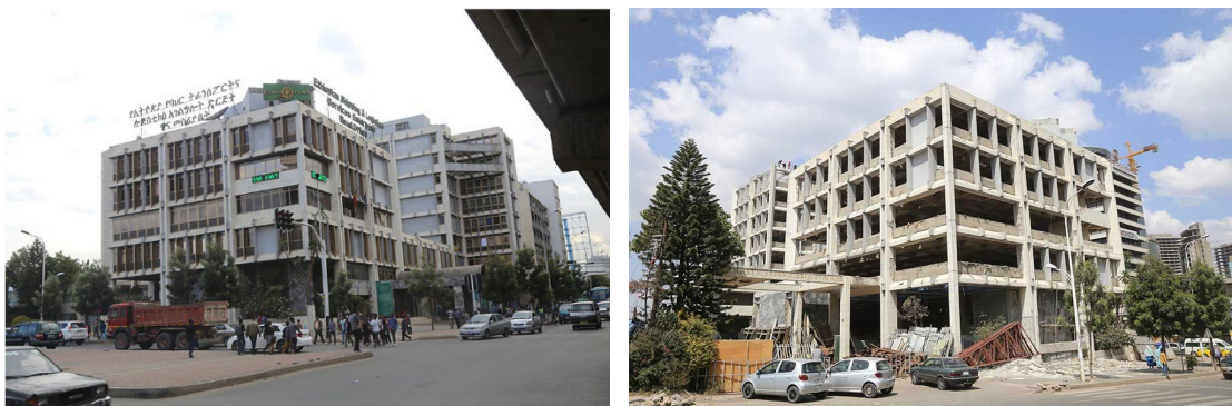
Figure 4-5 Before [Left] and After [Right] Demolition of Ethiopian Shipping Lines building in progress in 2019
