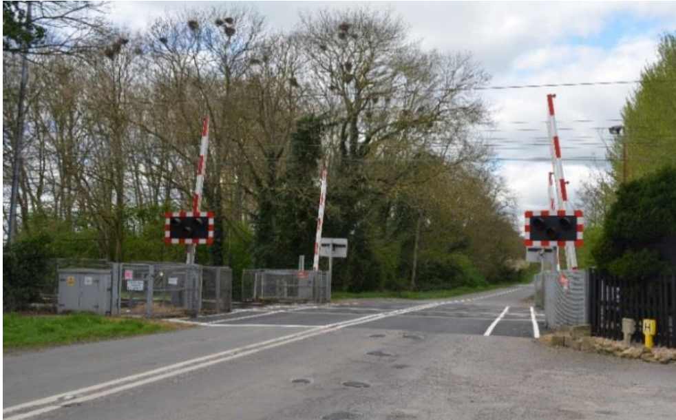
Figure 3-3: Carlton level crossing (MCB-CCTV)[47]
