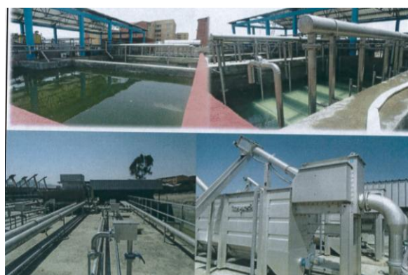
Bulbula, Mekanisa and Kilinto MBR wastewater treatment plant
