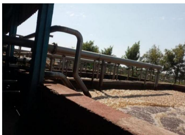
Membrane bioreactor wastewater treatment: Aeration tank
