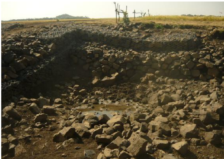
Plat 4. 5: Failure of sides made pond shrink
