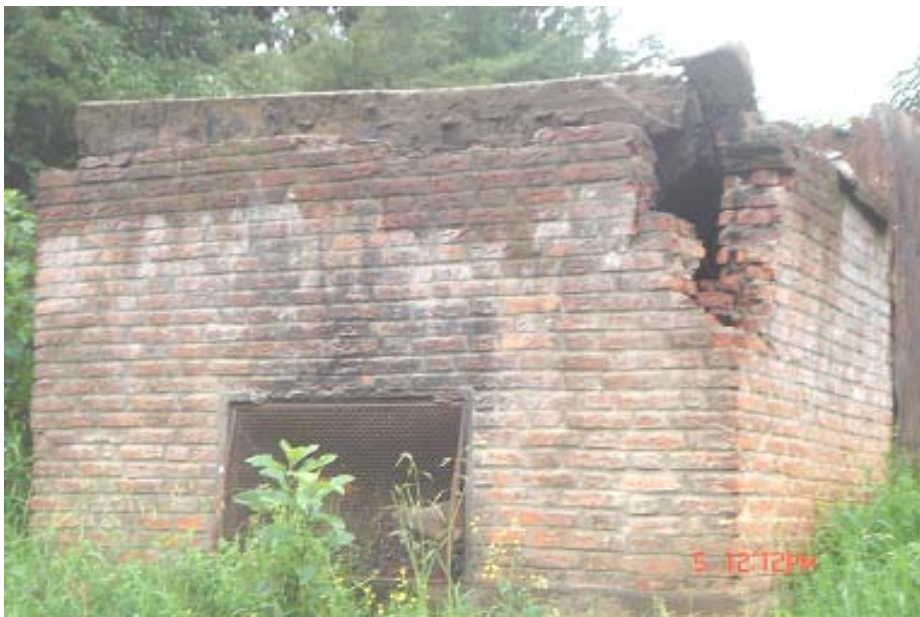
Figure 4.9 Damaged brick incinerator due to explosion from pressurized waste incineration
