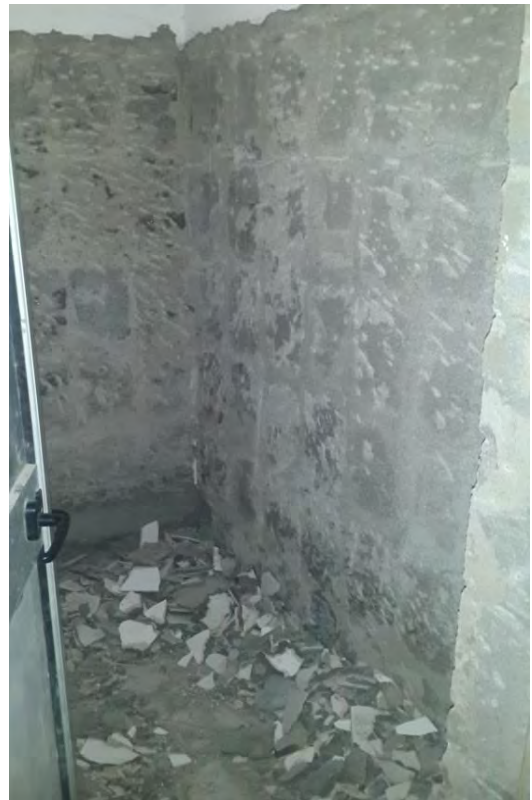
Fig 4.4: – Fallen ceramic wall tile
