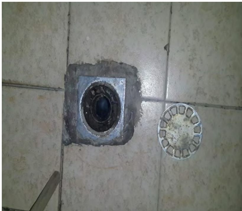
Fig 4.6: - Defective floor drain
