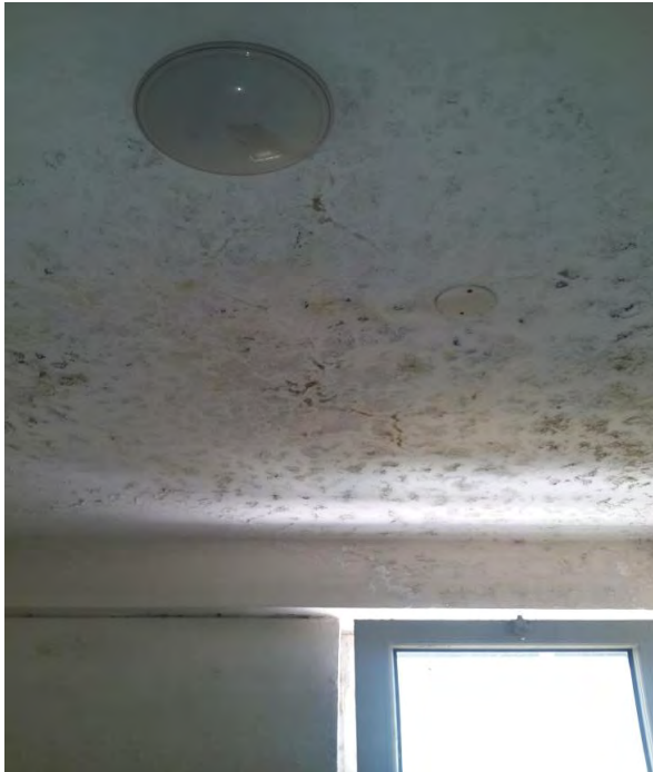
Fig 4.10: – Roof slab leakage
