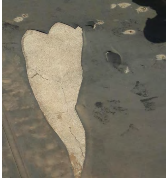
Fig 4.8: – Fractured water proofing membrane
