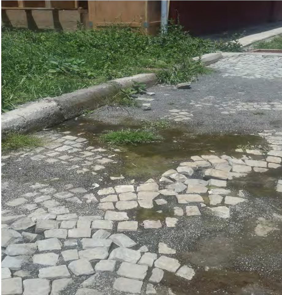
Fig 4.2: – Sludge drains to the surface
