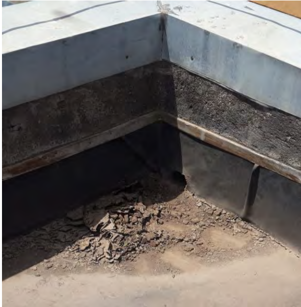
Fig 4.7: – dust accumulated at gutter opening
