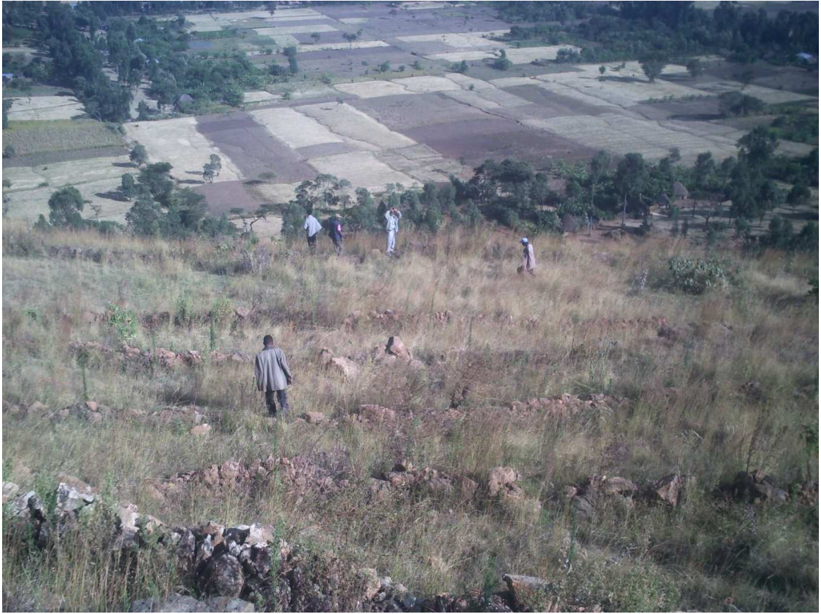
Fig.5.6 Stone bunds construct in Meles Zenawi memorial Park in Amburise Anijulo hillside. Source: field survey January 2014.
